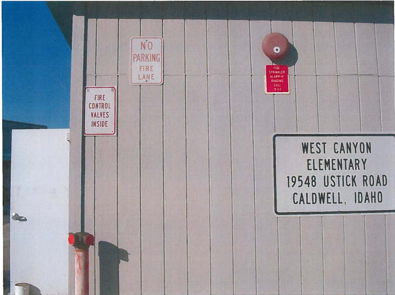
63-31132 License Exam 10/22/2010 Photo #5: Outside pump house main door facing west. Note two fire hose hookups in foreground of photo.
