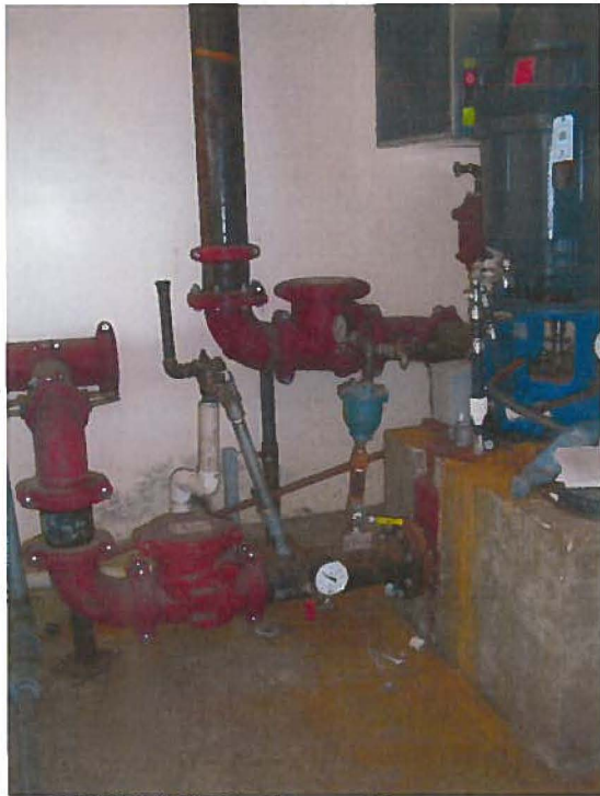
63-31132 License Exam 10/22/2010 Photo #2: Motor and well head on right. Lower discharge pipe 4 in dia. Discharge pipe out back of well underneath motor is 6 in dia pipe.
