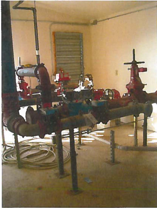
63-31132 License Exam 10/22/2010 Photo #3: Diversion system pipe lines. 4 in dia discharge pipe comes into this series of pipes from right hand side of photo. 6 in dia discharge pipe connects from above down pipe on far left hand side of photo. Individual lines for fire protection, irrigation, and domestic uses operated separately, but can be run together.
