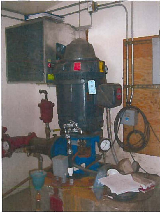
63-31132 License Exam 10/22/2010 Photo #1: US Electric motor (Serial # H060V2LG) mounted on well head. Note pressure gage in foreground.
