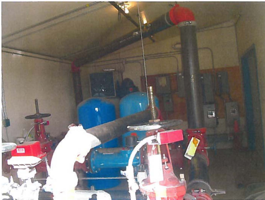
63-31132 License Exam 10/22/2010 Photo #4: Diversion system from doorway facing into pump house. Note flow meter in lower middle of photo on irrigation line.
