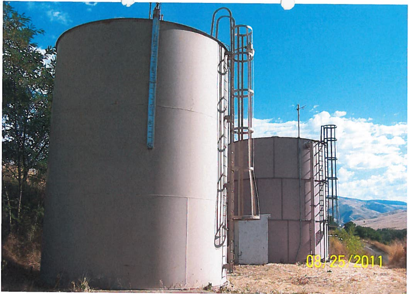
50,000 gallon + 65,000 gallon storage tanks
