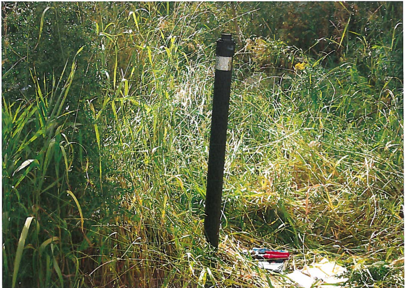
Vertical pipe at Spring
