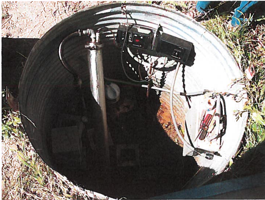
Figure 5: Solar pump system
