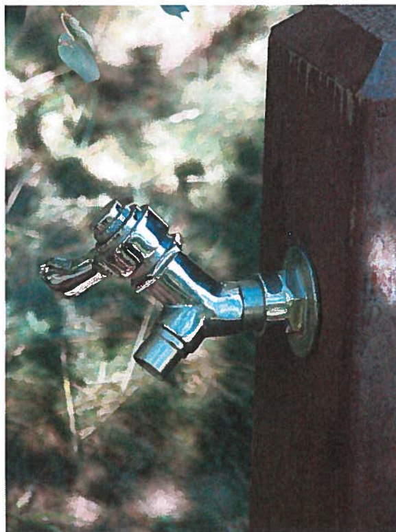
Figure 6: Threadless spigot installed at campgrounds
