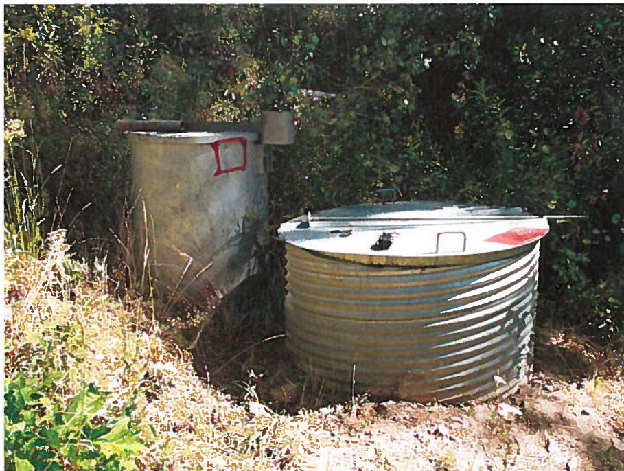
Figure 4: Hatch for 5000 gallon storage tank and housing for chlorinator
