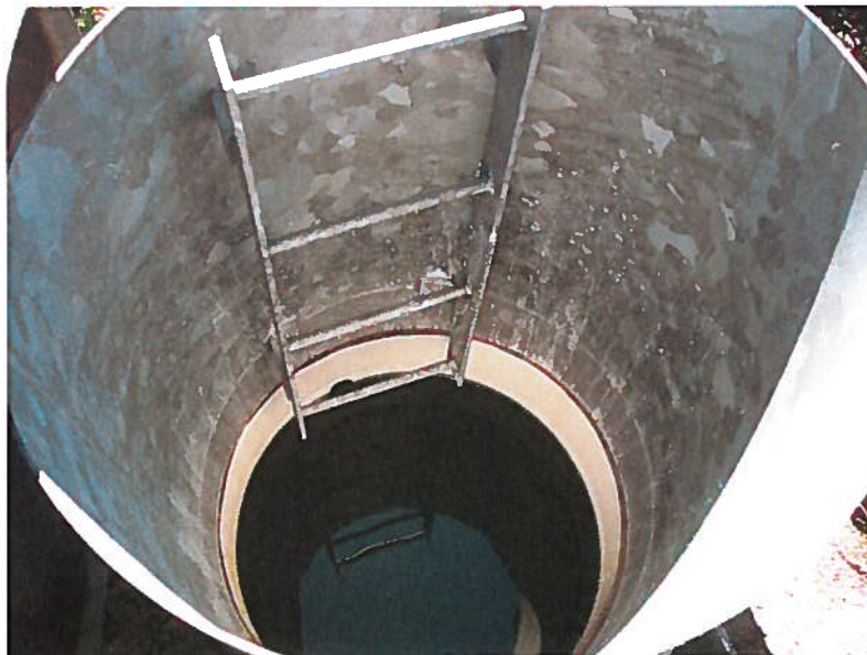
Figure 6: Looking down hatch into 15,000 gallon storage tank
