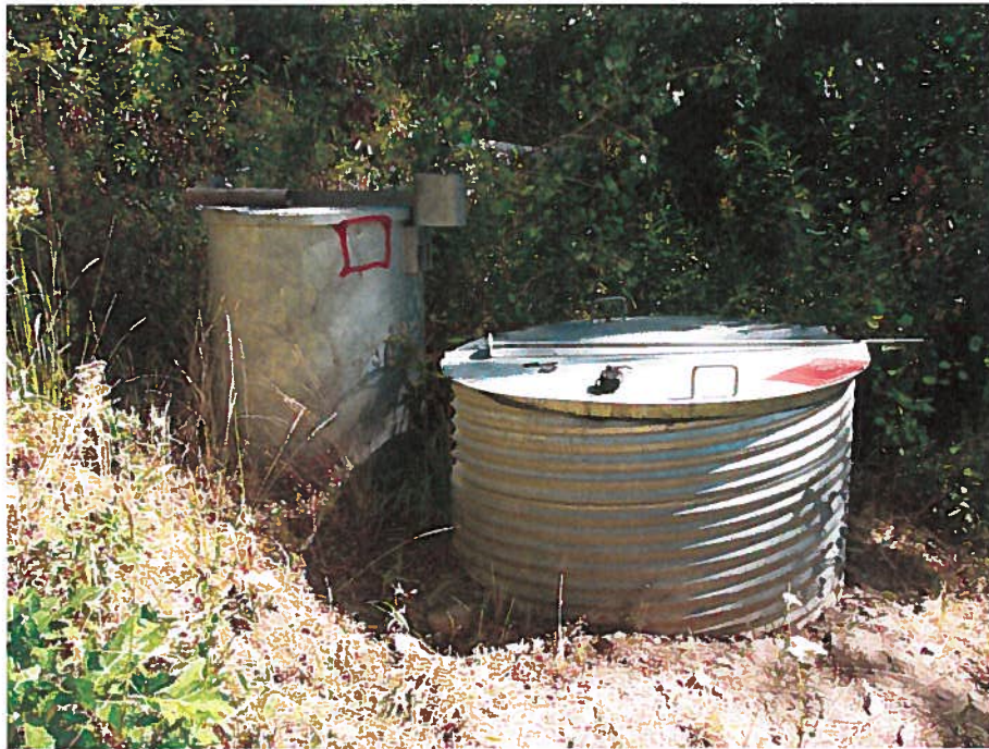
Figure 3:Hatch for 5000 gallon storage tank and housing for chlorinator
