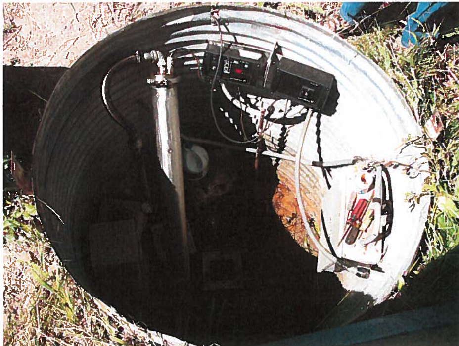
Figure 4: Solar pump system
