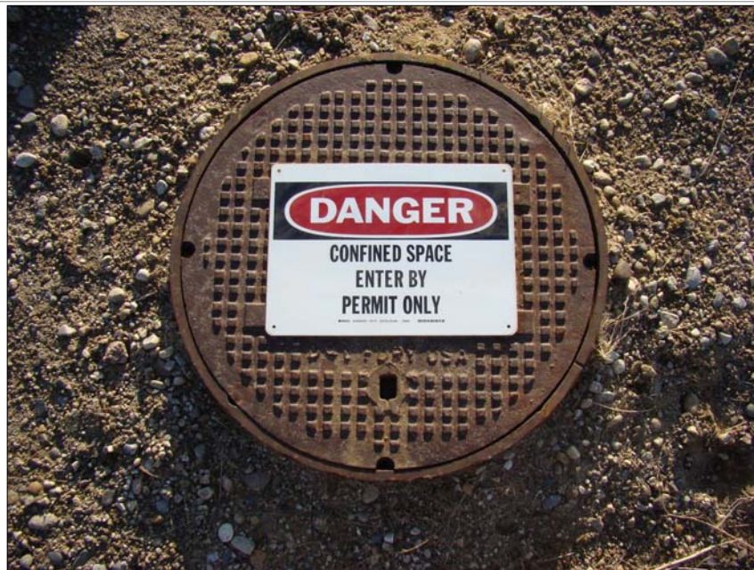
Manhole entrance to ISCI Well #7 plumbing vault.
