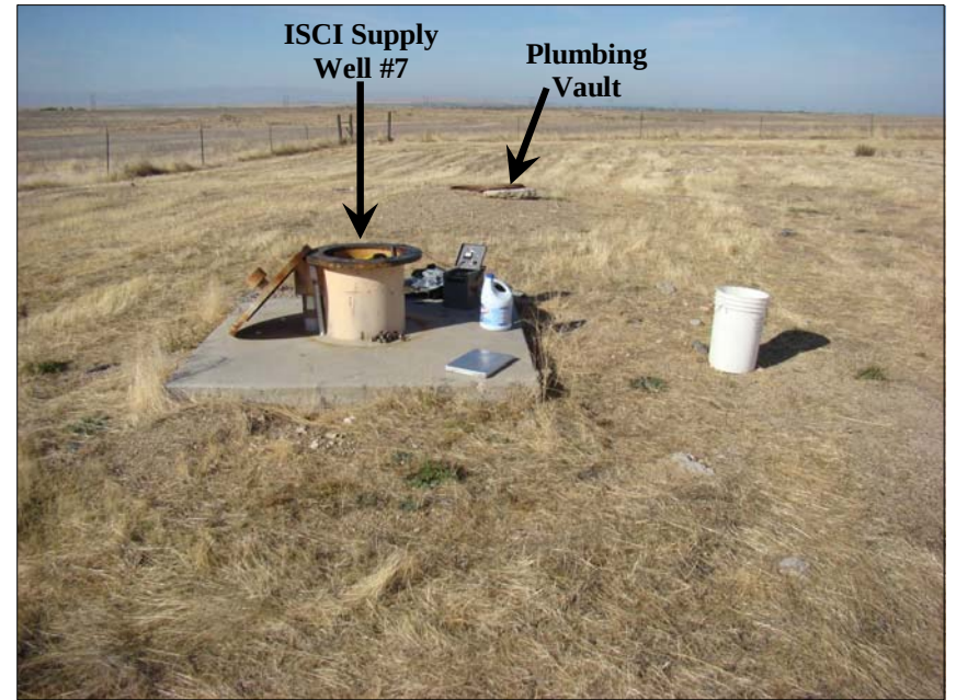
View looking west at ISCI supply Well #7 with lid removed for water level measurement during the pump test.
