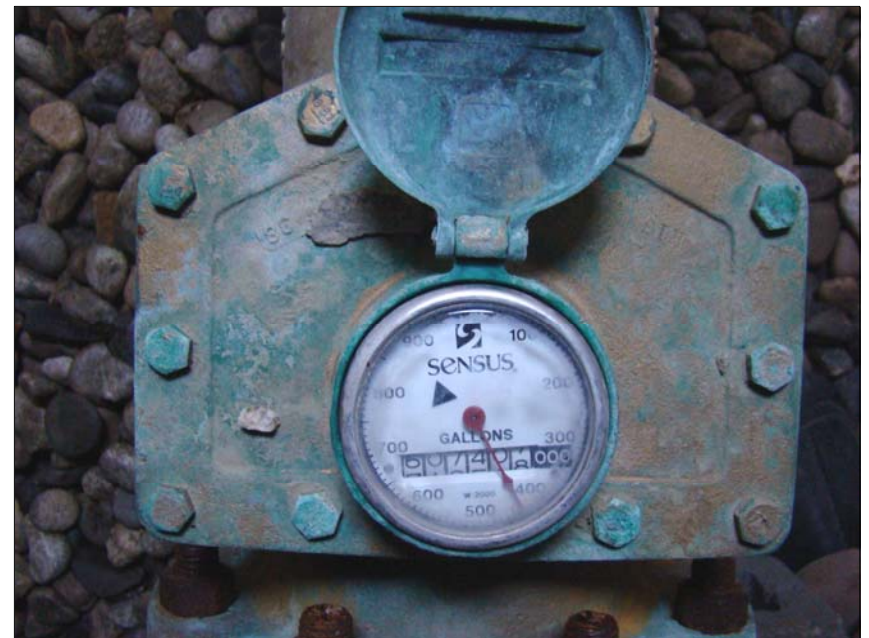
Totalizing flow register on 8-inch Sensus flow meter for ISCI Supply Well #8.
