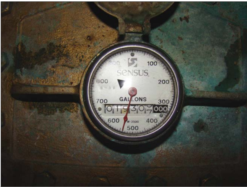
October 13, 2011 photograph of the totalizing flow register of the 8-inch diameter “Sensus” flow meter for ISCI Supply Well #7 (ICC Well #2). Flow is measured by timing of rotating needle = 1,000 gpm per rotation.
