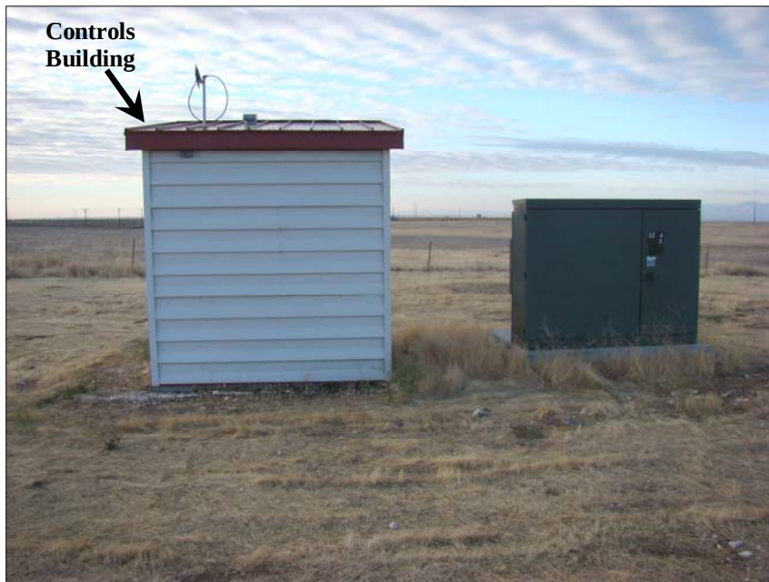
South-looking view of ISCI Well #7 electrical control house and power transformer.
