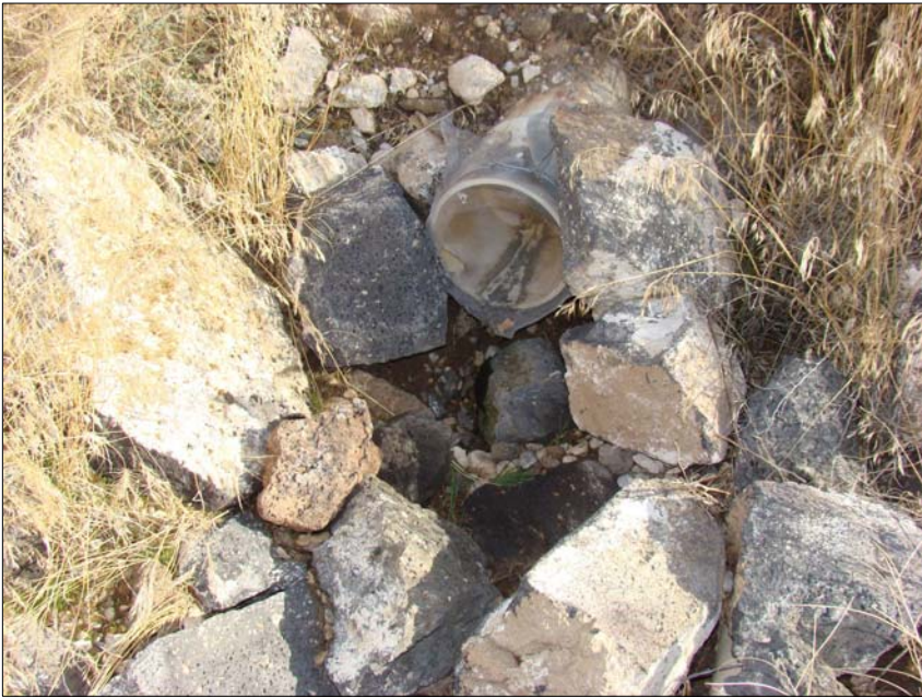
View of 8-inch diameter PVC flush-line day-lighting approximately 120-feet from ISCI supply Well #7 plumbing vault.
