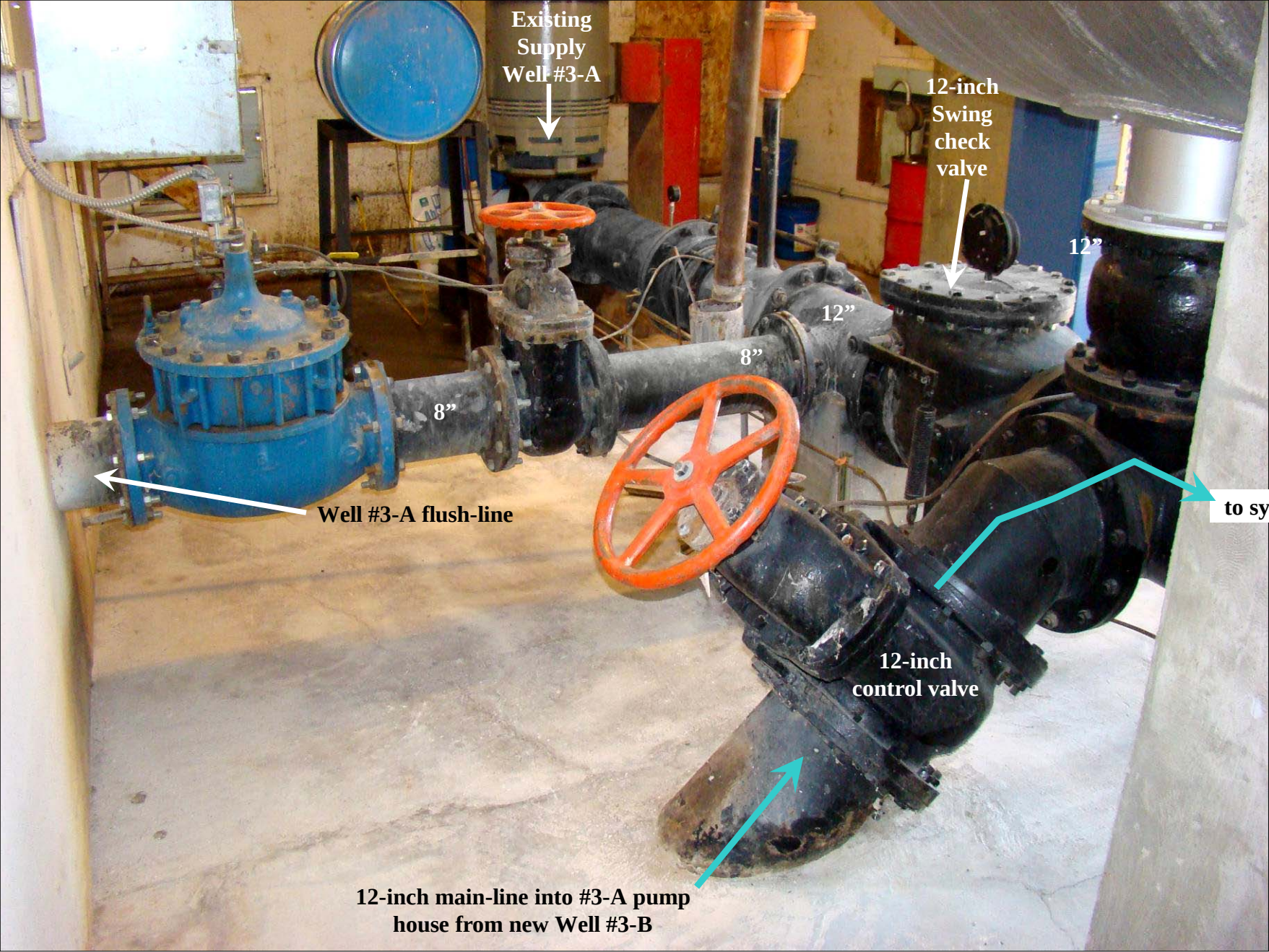
Figure 10. Photo of the 12-inch main from new replacement Well #3-B entering plumbing in ISCI supply Well #3-A pump house.
