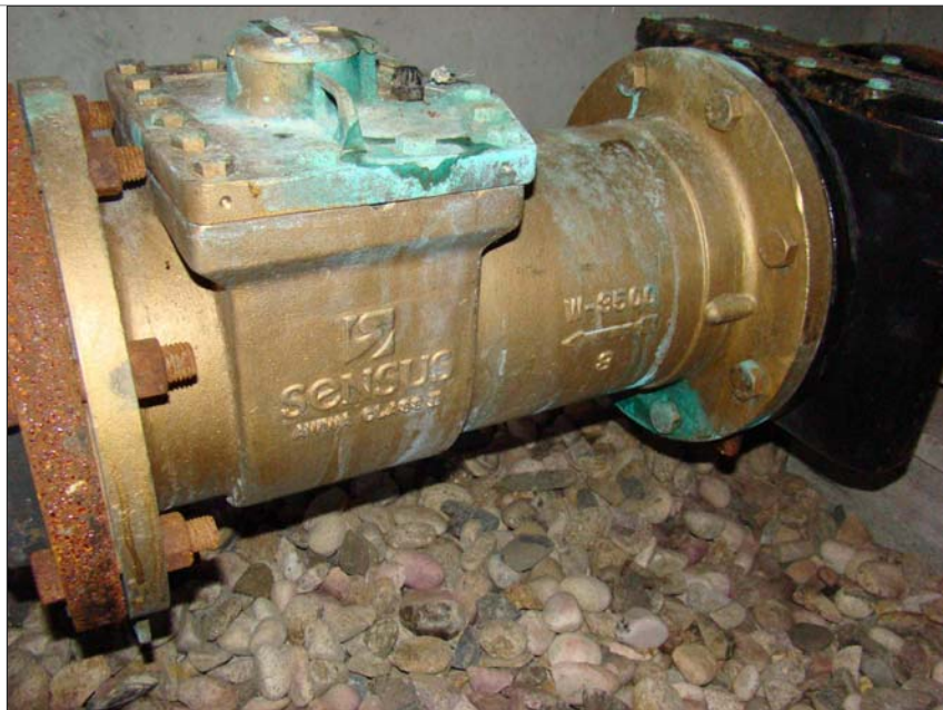
8-inch Sensus flow meter with integral flow-straightener (Model #W-3500 and Serial #1558270) installed in ISCI Supply Well #7 plumbing.
