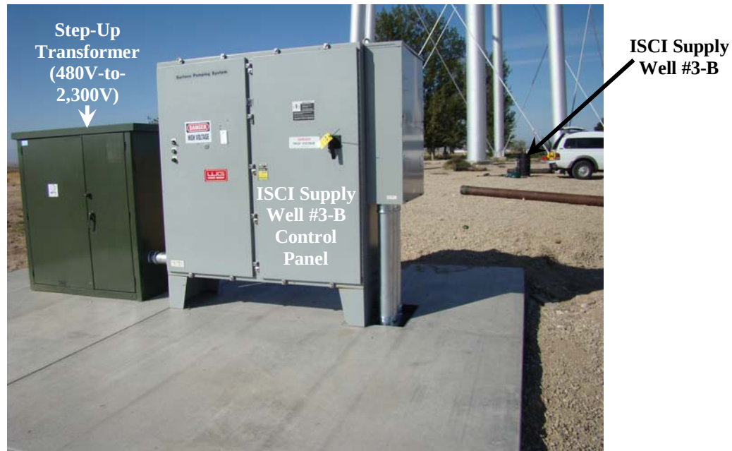
Photo looking west at power supply for ISCI Supply Well #3-B.
