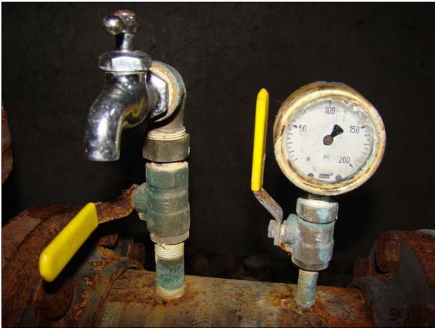
October 13, 2011 photograph of water quality sample tap and main line pressure gage (broken) on the ISCI Well #8 (ICC Well #1) well head plumbing.
