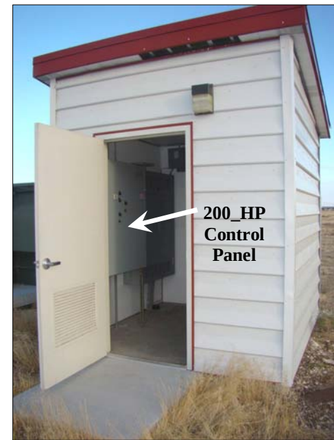
View of the inside of ISCI Well #7 (ICC Well #2) controls building looking at the 200-HP control panel for the submersible pumping plant.
