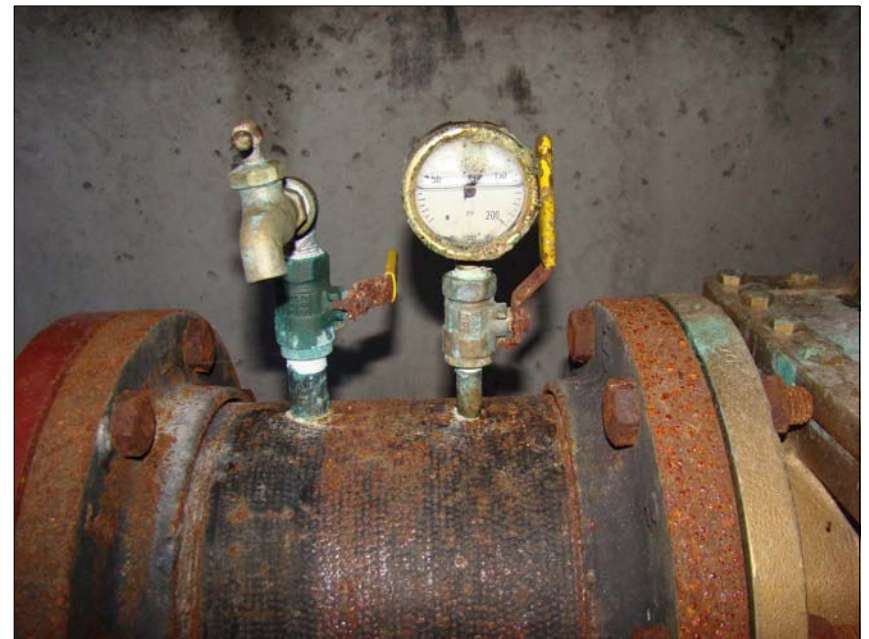
Water quality sample tap and main line pressure gage (broken) in the discharge piping of the ISCI Well #7.
