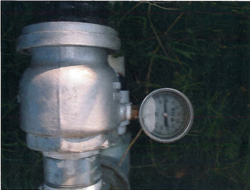
Pressure gage – running at 34 psi (Permit holder had sprinklers running on native grasses)
