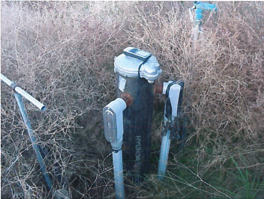
Picture of Well head – submersible pumps in well
