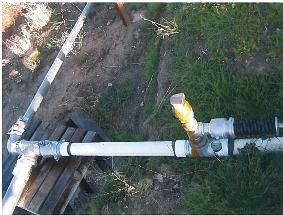
Location sprinkler system is currently operated from – Note pressure gage and pipeline
