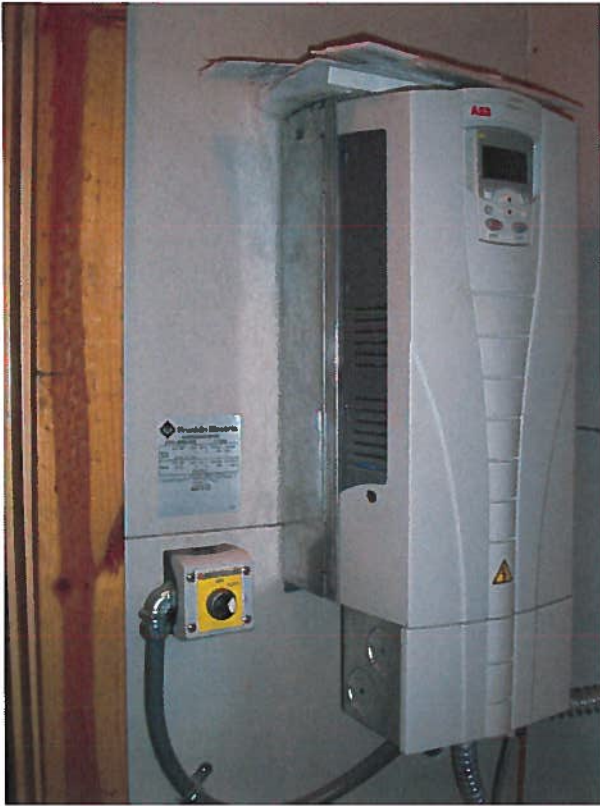
Well pump control box. Motor info sticker on wall inside house basement.
