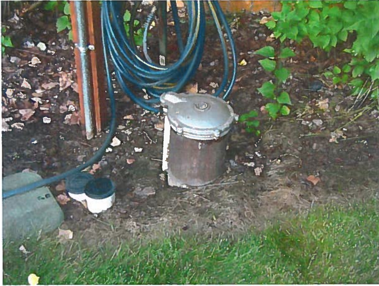
Photo 1 – 8” well behind home at NW edge of property.
