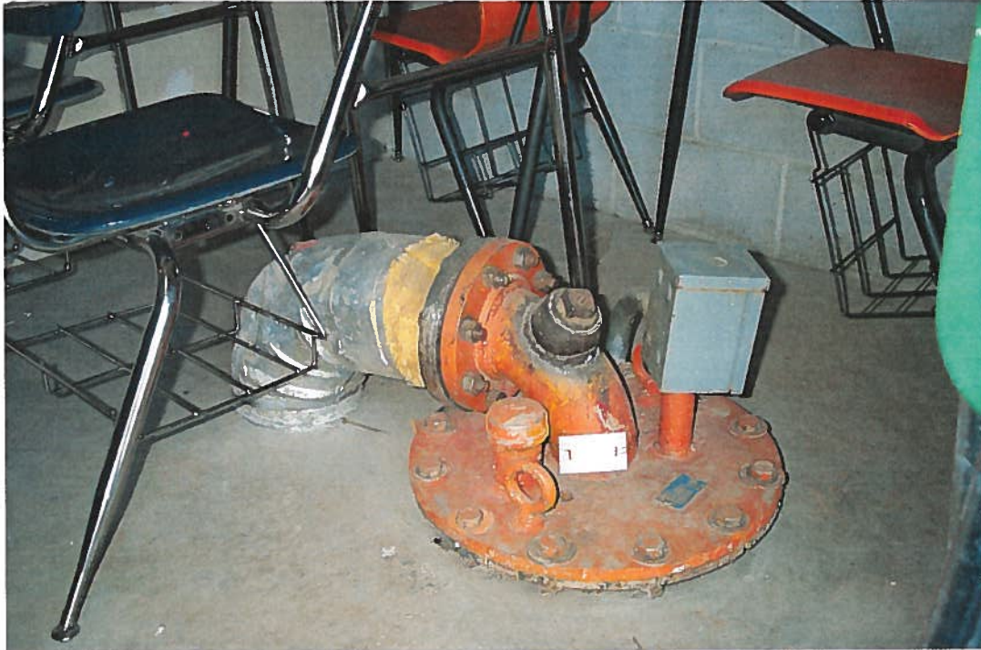
Geothermal Well At High School
