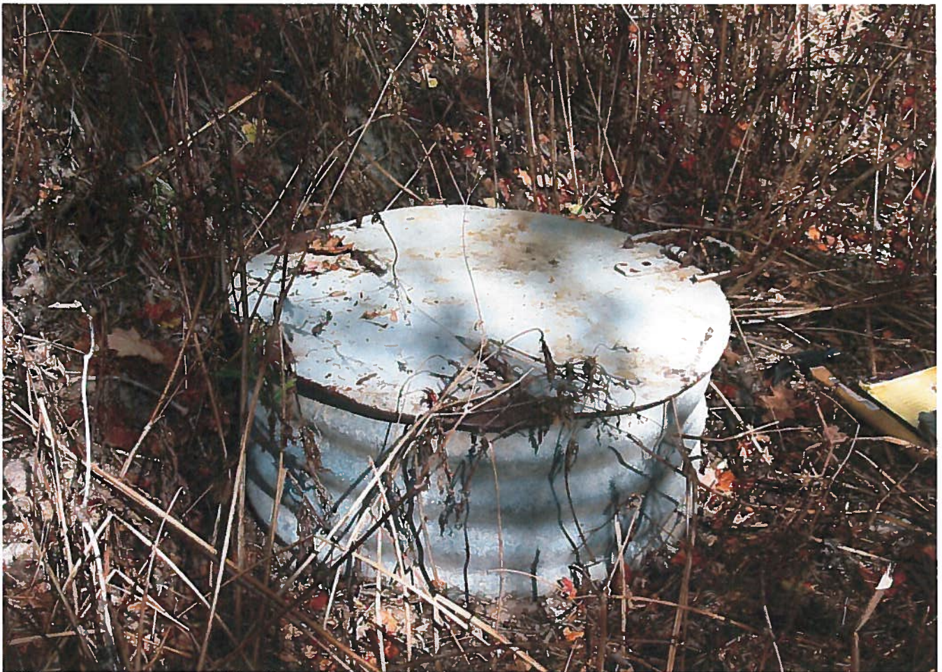
POD - outlet of cistern
