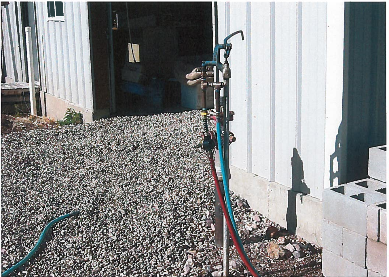
Hydrant at shop
