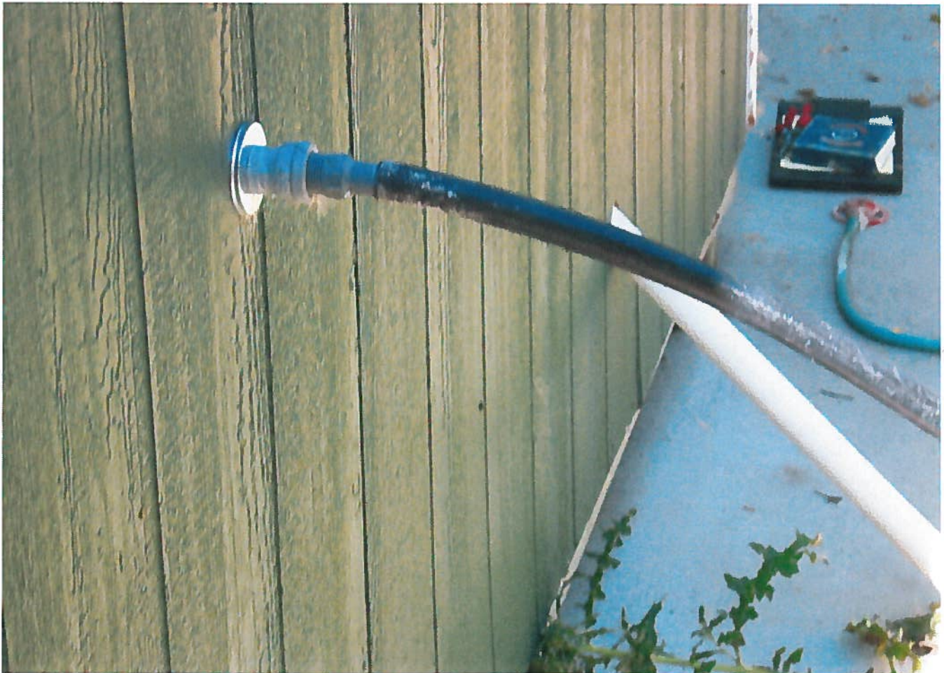
Water Pipe Entering Gunnell Cabin
