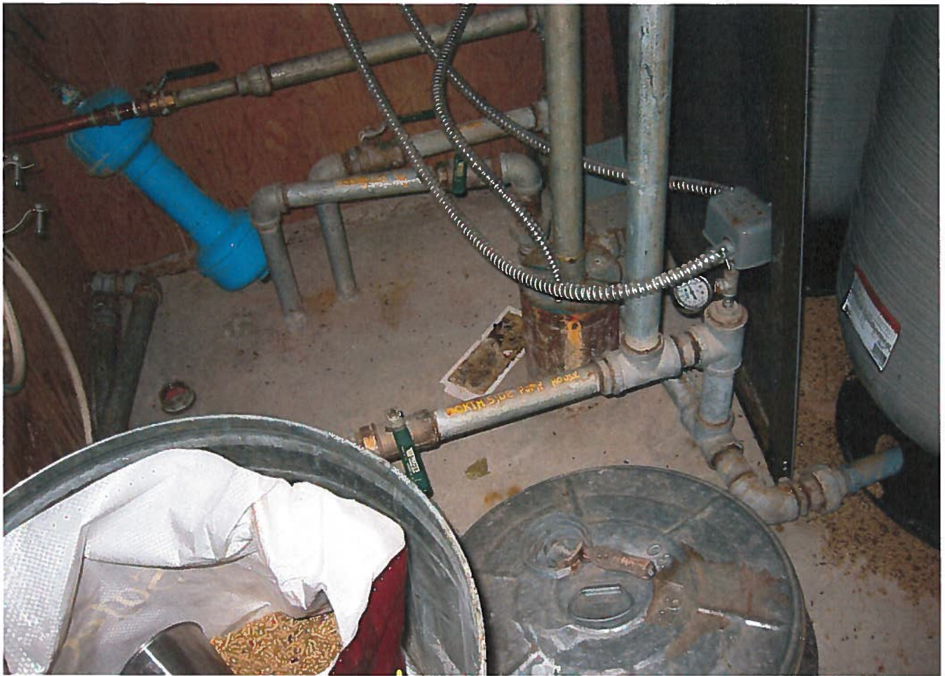
Wellhead and plumbing in well house.
