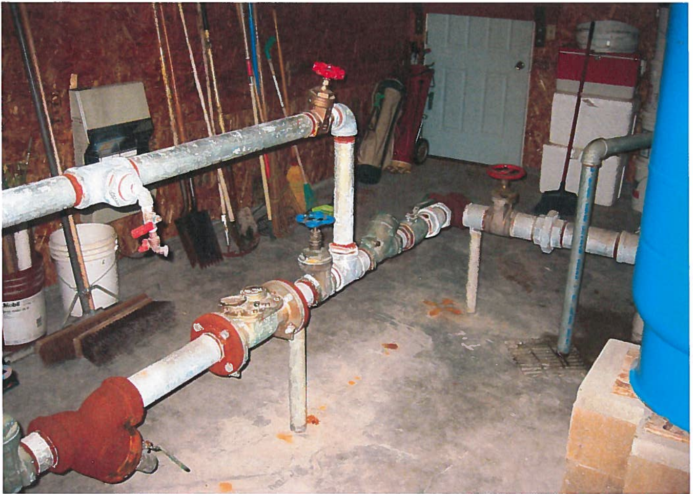
Plumbing inside well house.
