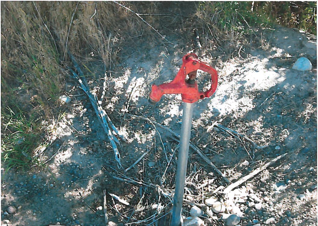
Hydrant on Empty Lot
