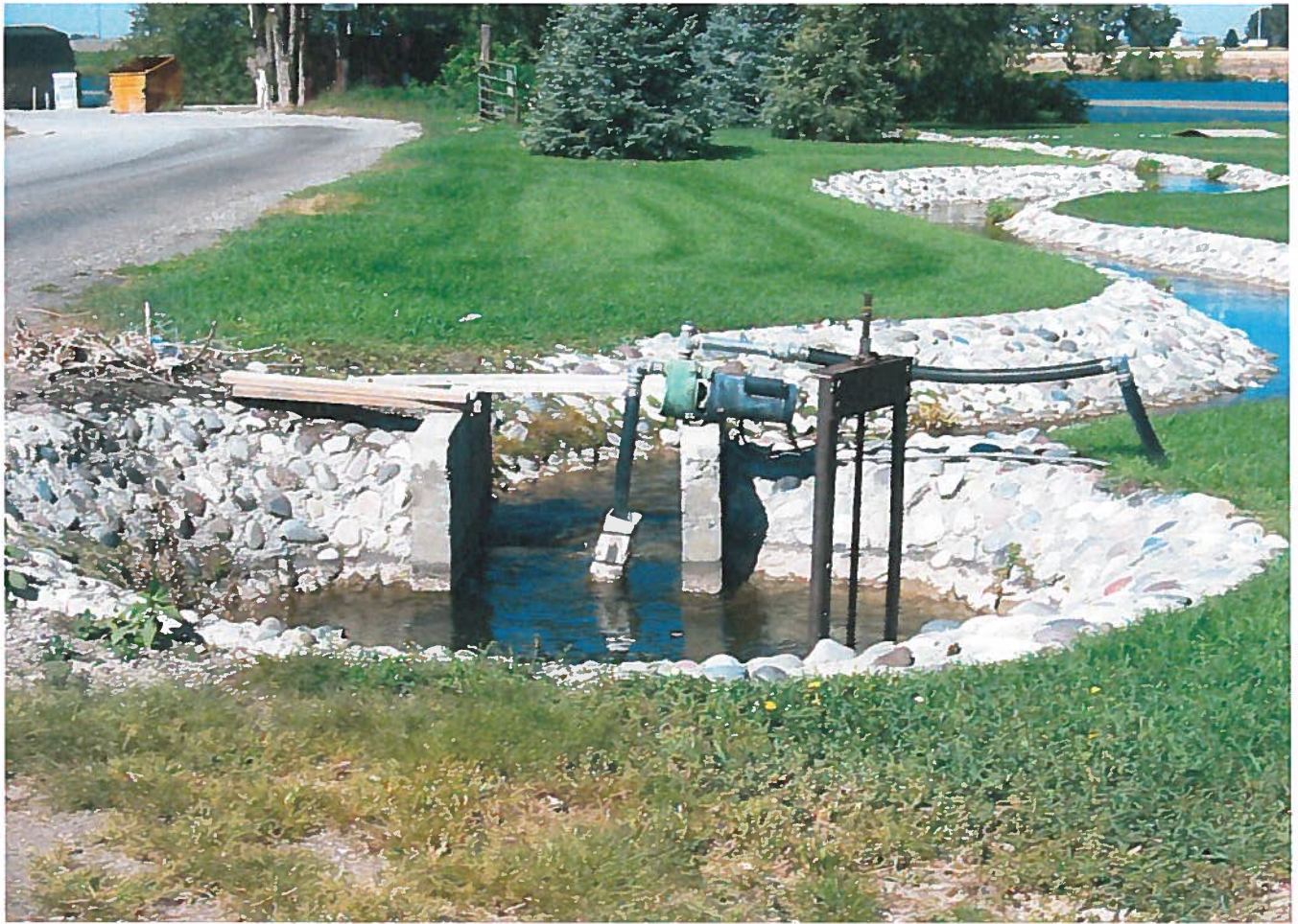
Canal water being pumped for Outside use in subdivision
