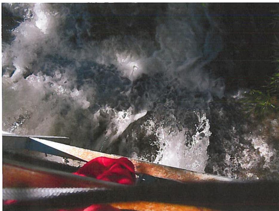
63-12304 License Exam 7/15/2010: Looking down from on top of downstream weir/check at leakage on west side of check. Far right side of weir crest extreme left in this photo.
