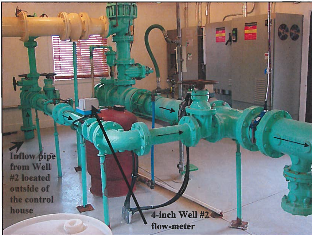
January 25, 2010 photograph taken inside the Kuna Danskin well house showing the discharge piping from the Danskin Well #2 located outside the building
