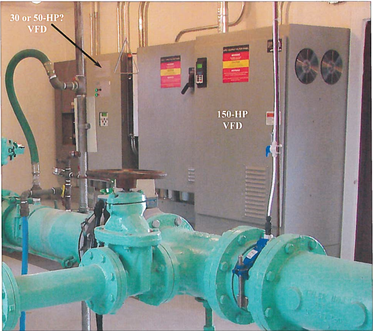
Figure 10. Photos of the VFD drives for the Danskin Supply Wells and Danskin #1 150-HP Motor Tag
