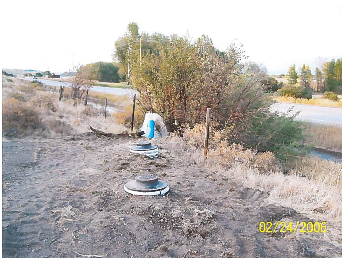
Terminus of the Sam's Hollow mitigation pipeline.
