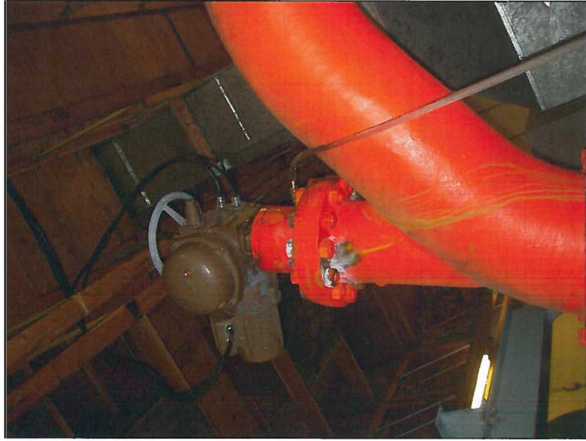
Picture 16 – control motor for needle valve of the upper penstock line.
