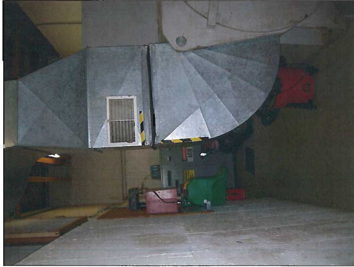
Picture 20 – power house generator exhaust system.
