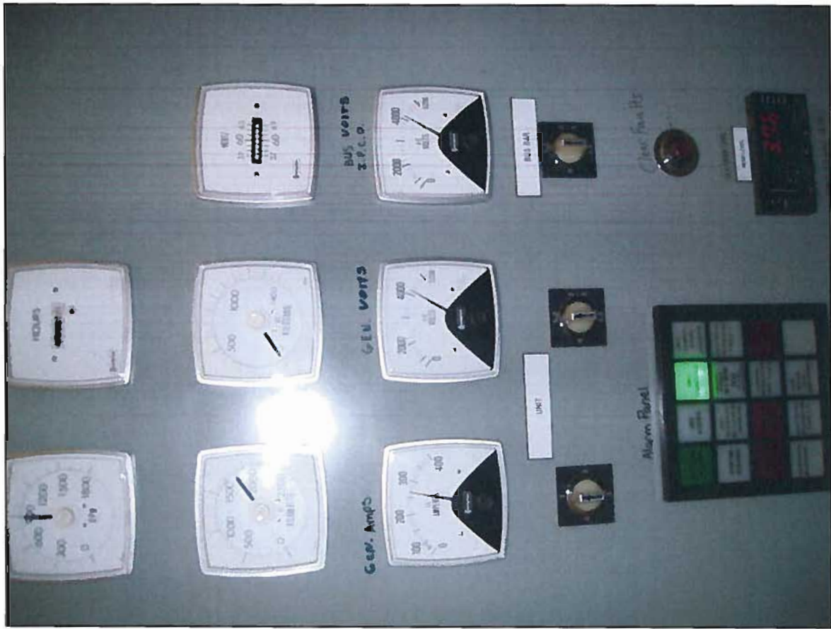
Picture 23 – control system readouts.
