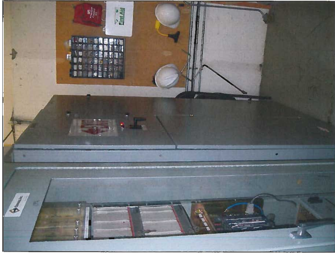
Picture 22 – power plant control system.
