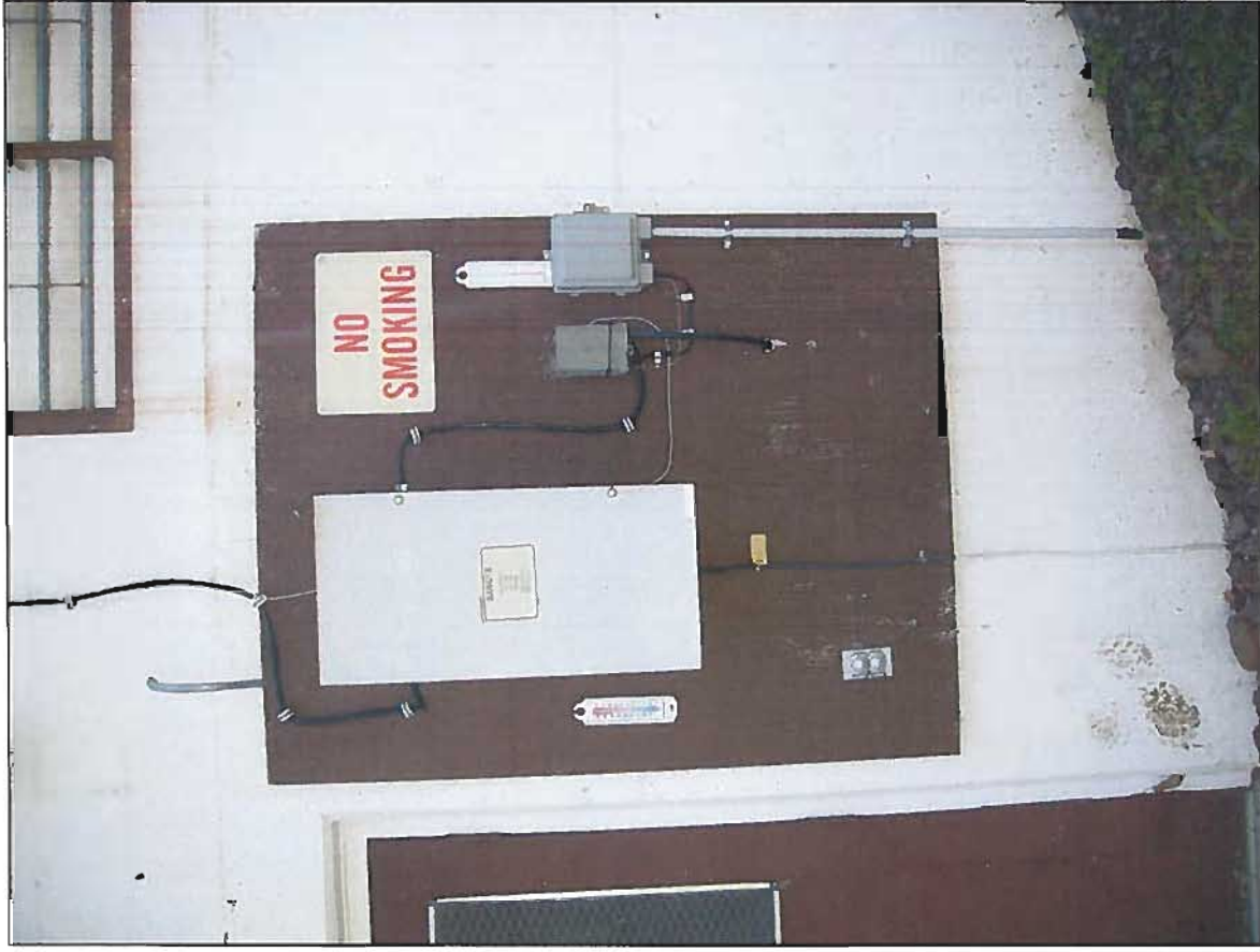
Picture 13 - entrance and main exterior electrical breaker box of power house (west face).
