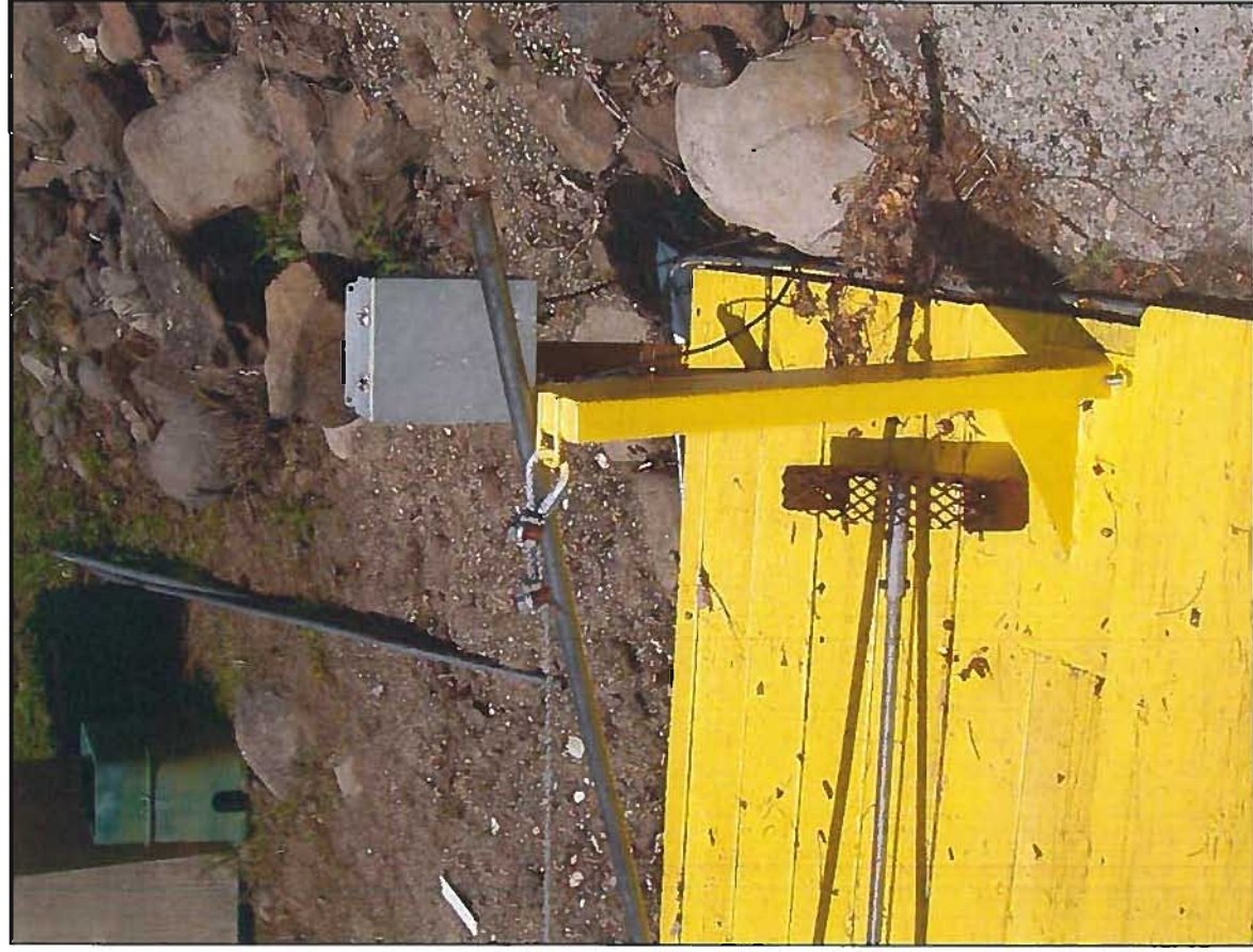
Picture 8 - photo of pressure transducer that measures head over the penstock inlet (northeast corner of platform).
