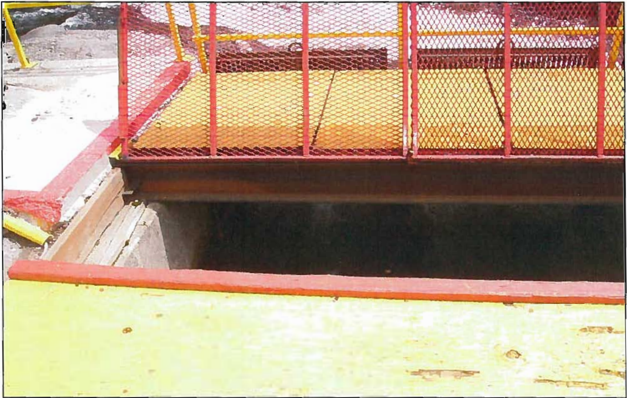
Picture 3 – photo of two of three slide gate intake devices, looking upstream with Elk Creek in background.
