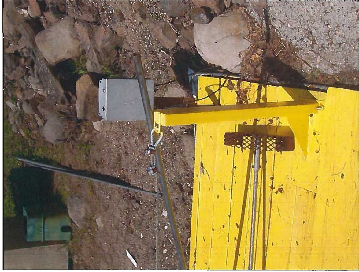
Picture 8 - photo of pressure transducer that measures head over the penstock inlet (northeast corner of platform).
