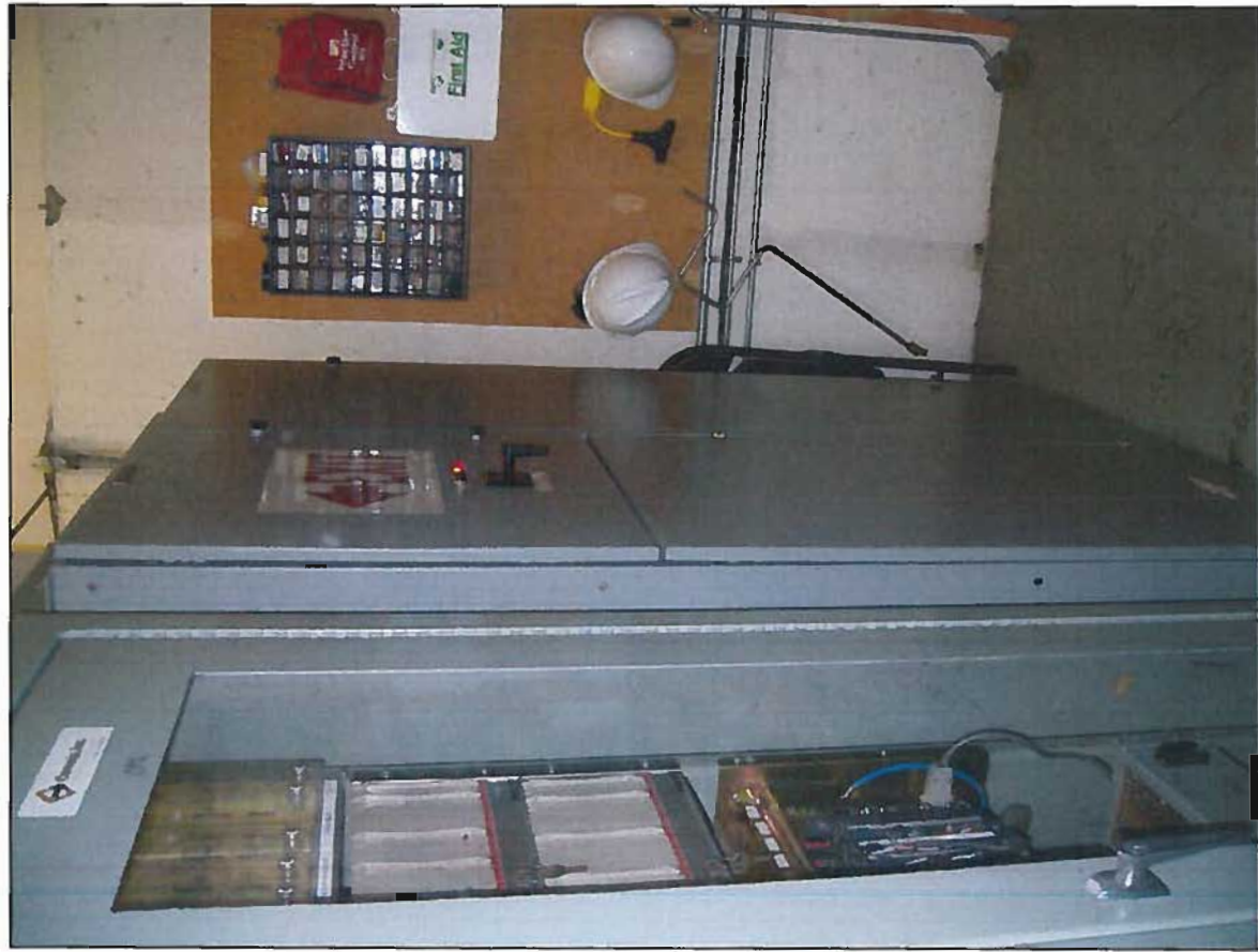
Picture 22 – power plant control system.
