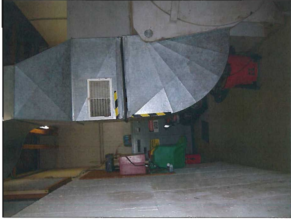
Picture 20 – power house generator exhaust system.
