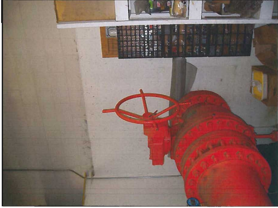
Picture 14 – entrance of penstock into power house. Gate valve fitting allows for the isolation of the turbine. Note pressure gage located just upstream of the division of the penstock into two separate lines (division not shown)
