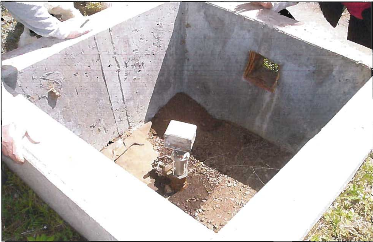
Picture 10 – photo of meter vault and non-functioning meter display.
