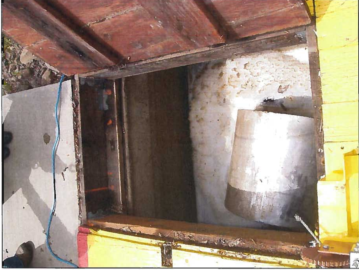
Picture 9 - photo of inlet to penstock (below water line) note the float device use to control flow into the penstock. The penstock intake is located in the northwest corner of the platform.
