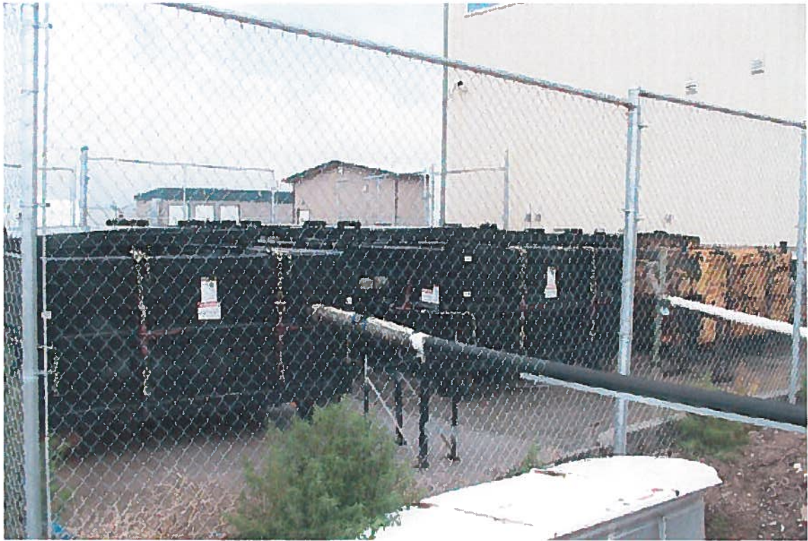
Wastewater Pipe exiting settling tanks
