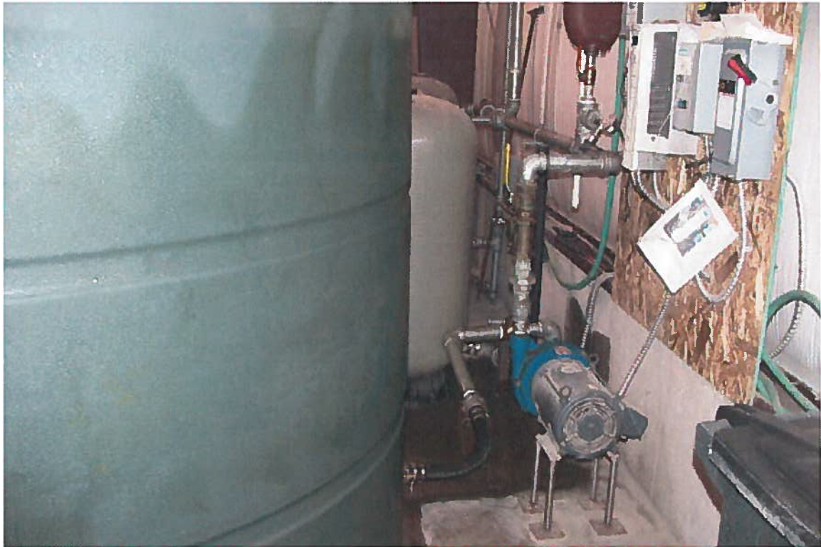
Booster Pump and inside plumbing
