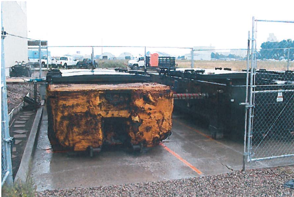
Sediment settling tanks
