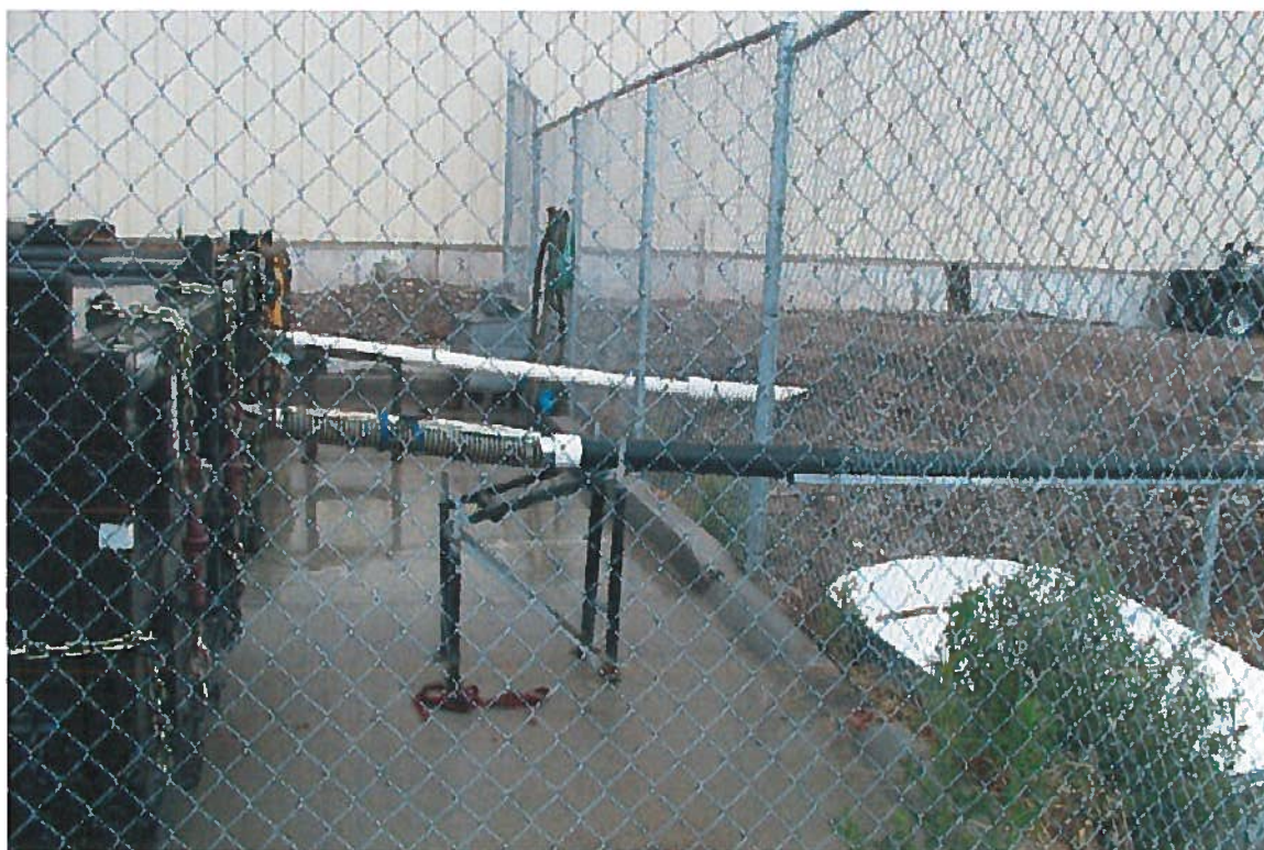
Wastewater pipe exiting settling tanks
