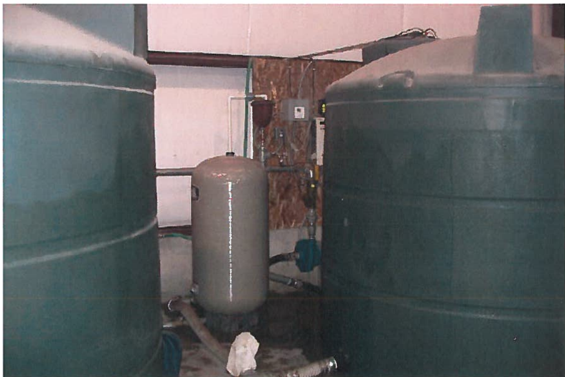
Pressure and holding tanks
