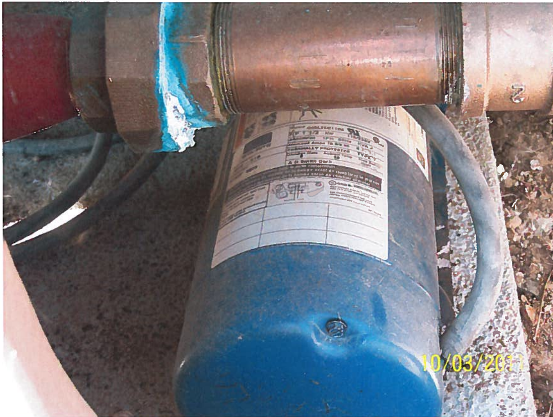
Pump inside the pump house
