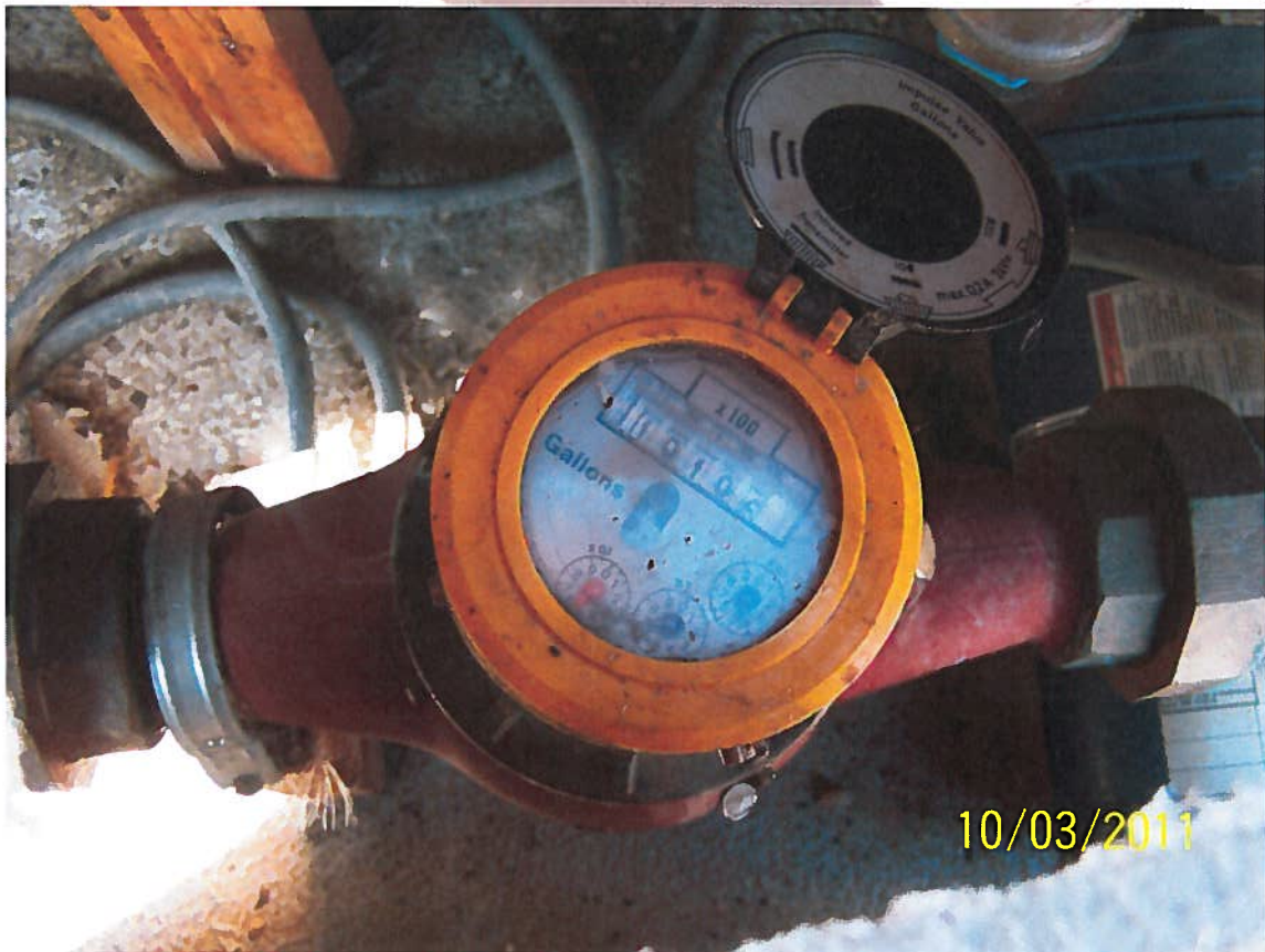
Flow Meter within pump house
