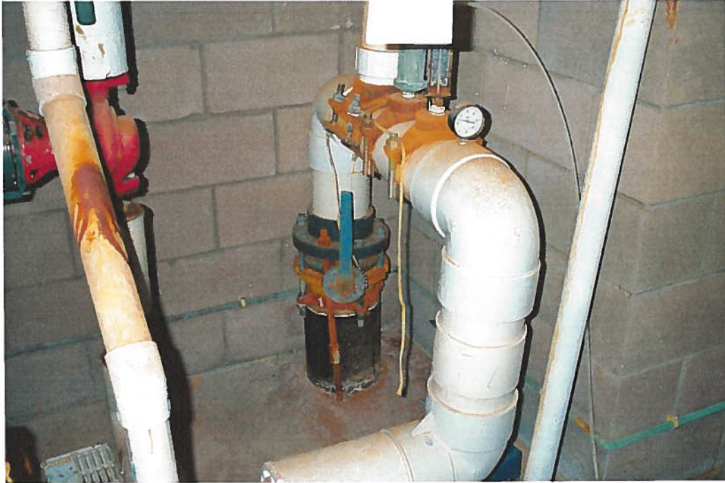
Pipeline Carrying Geothermal Water Into Pool Building
