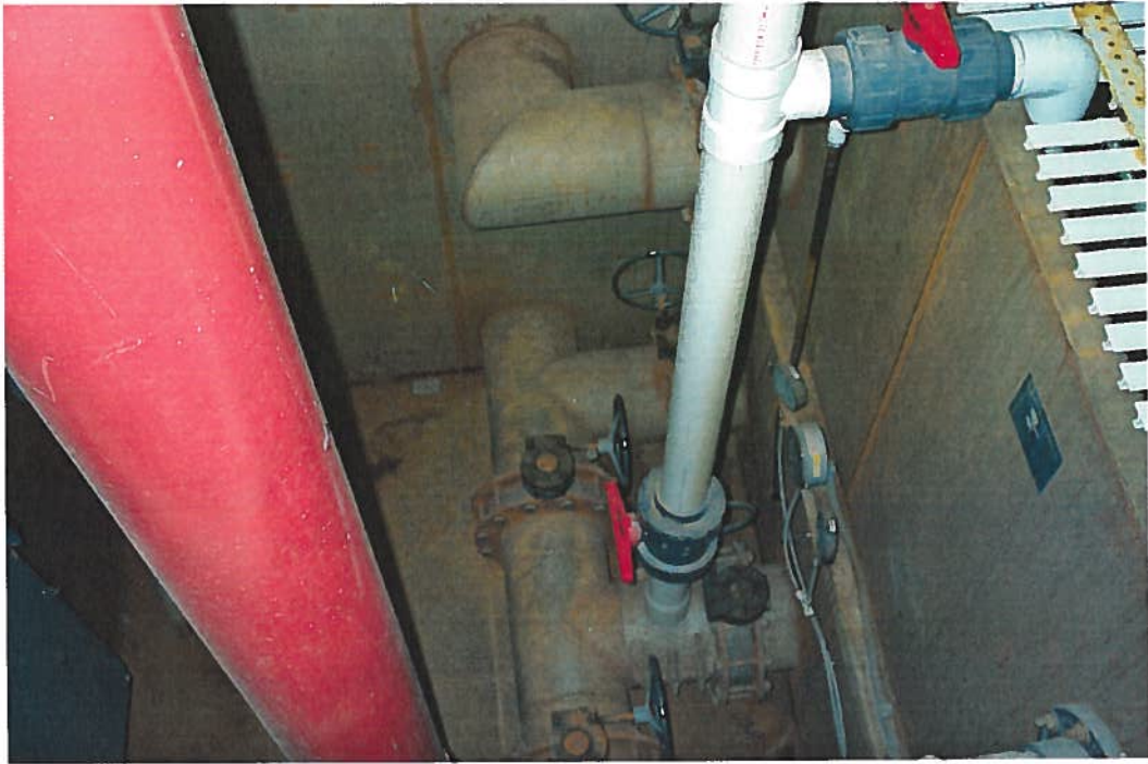
Pipeline Carrying Geothermal Water To Pool
