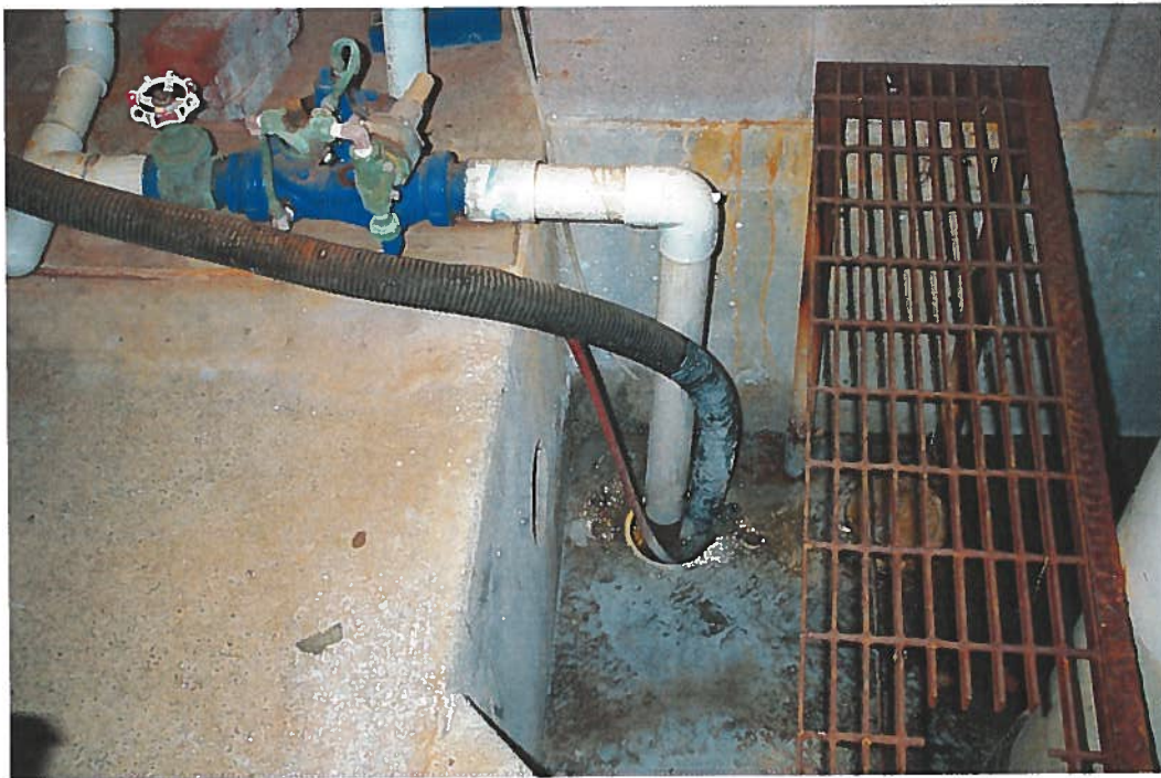
Overflow Carrying Excess Geothermal Water Into Sewer System
