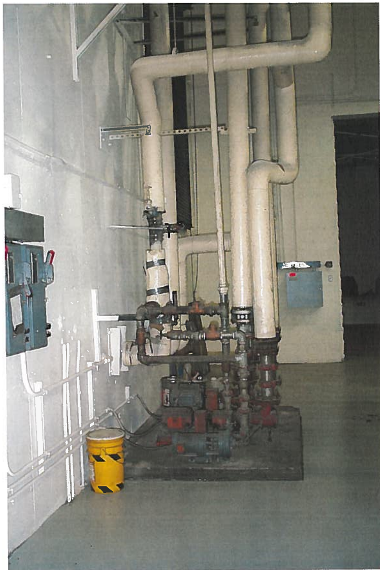
Pressure Pumps & Pielines Carrying Geothermal Water to Sawtooth School & Twin Falls City Pool
