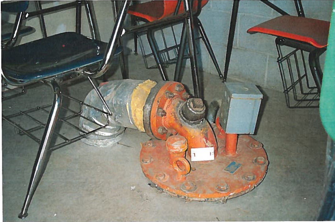
Geothermal Well At High School
