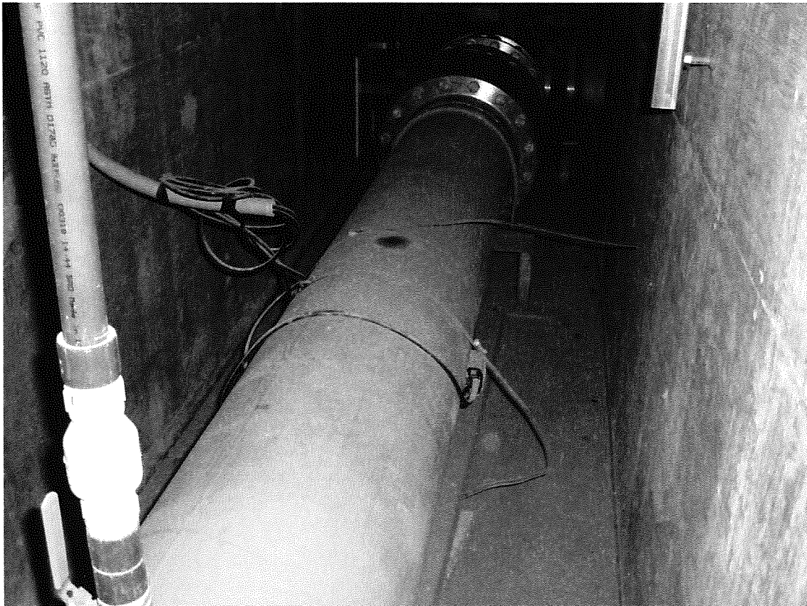
Well 5 ultrasonic flow meter
