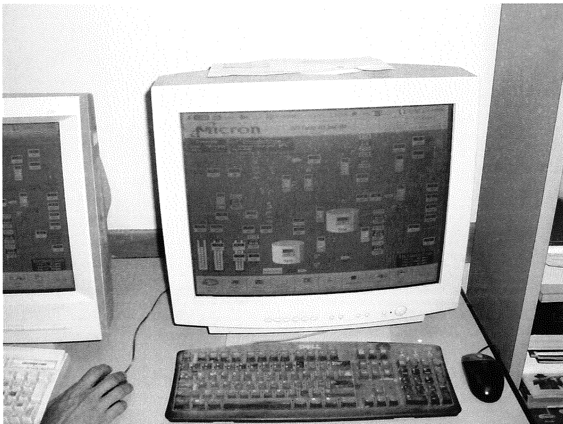
SCADA system screen in Building 22
