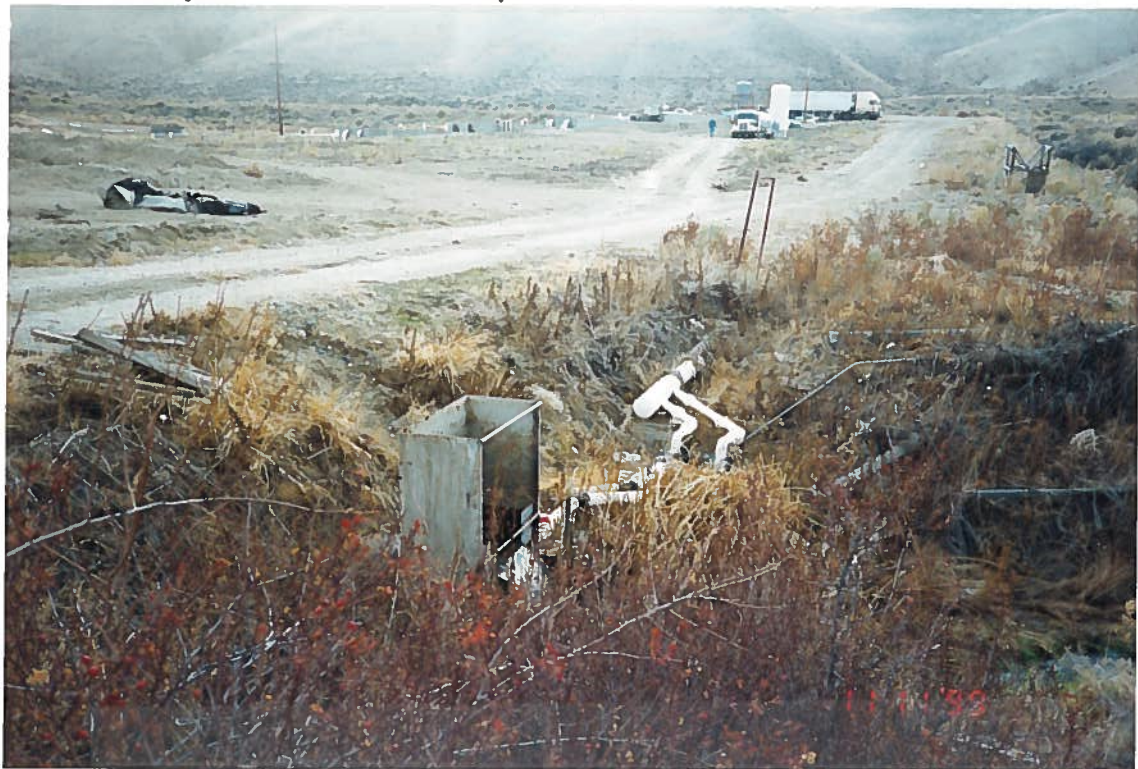
Measuring Device & Re-lift Pumps on Warm Creek Below Settling Pond
