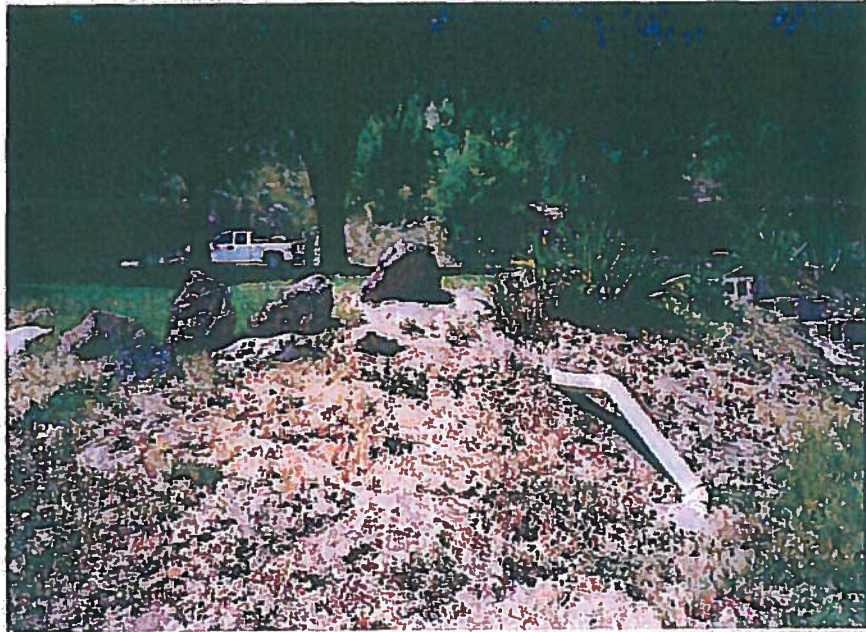
Downstream collection box with overflow pipe to river. Permit # 29-7936
