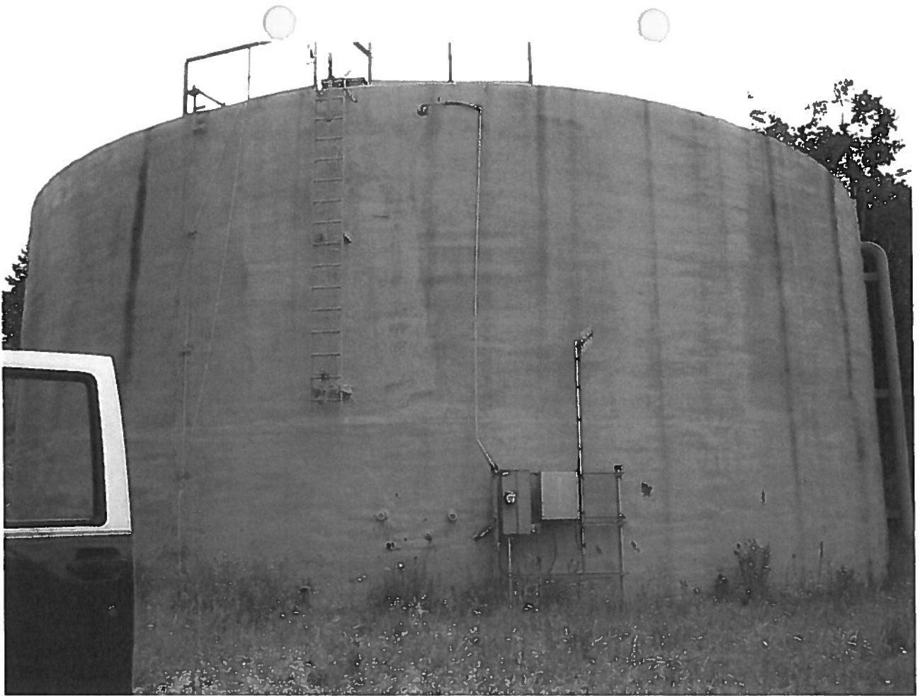
500,000 gallon storage tank
