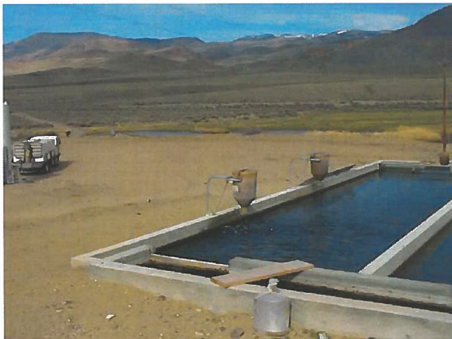
Below: Hatchery raceways in foreground, settling pond in background. Re-lift pump in middle and left side of photo near road.
