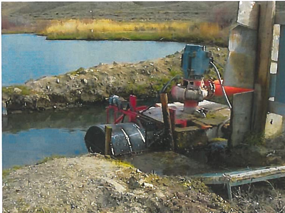
Top: Luper re-lift pump and settling pond.
