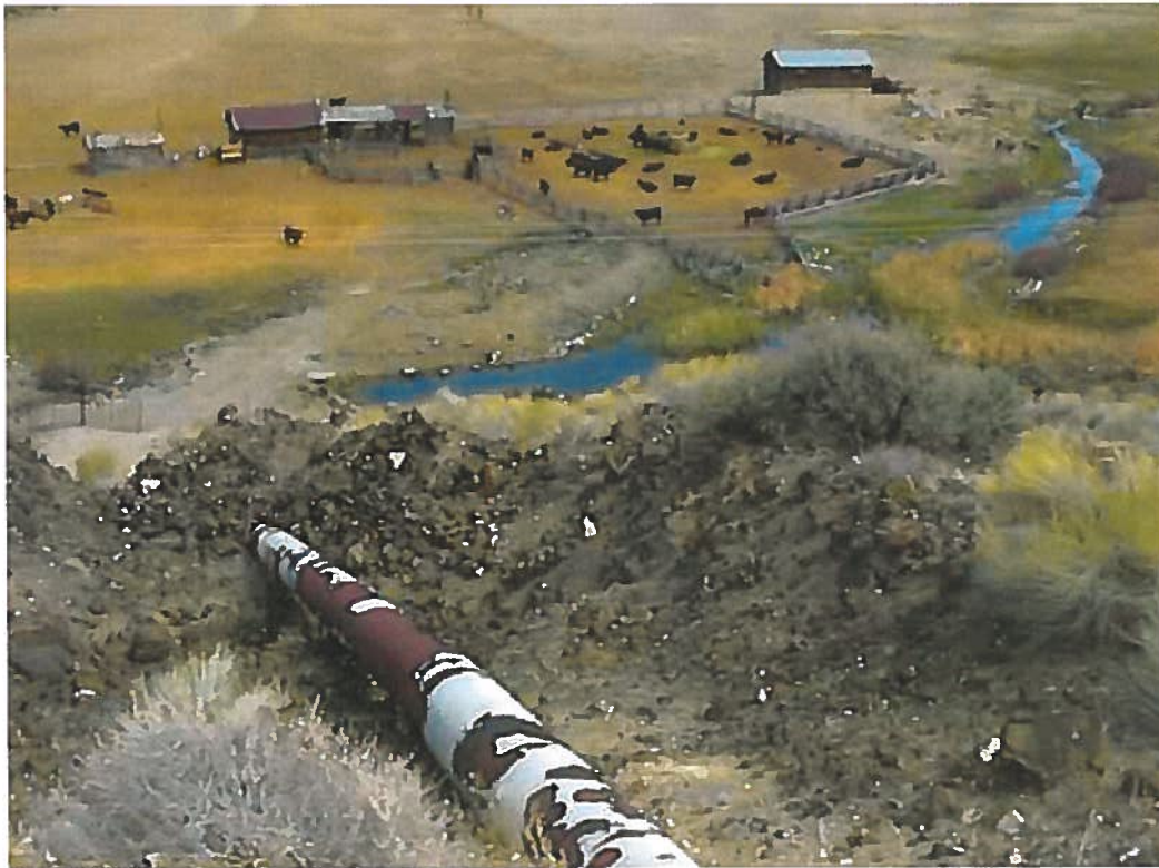
Above: Morganroth re-lift pumpline from re-lift pump in creek to canal. Warm Spring Creek in background. Pump not visible in photo.
