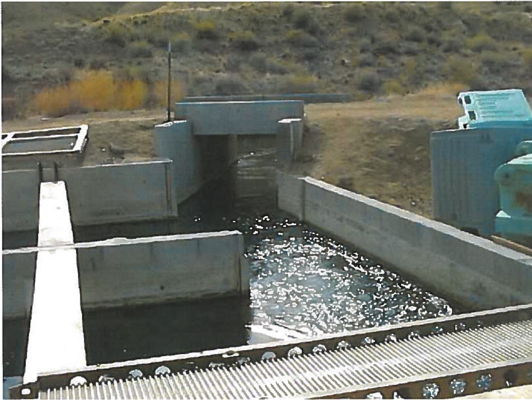
Top: Lupher tailrace and discharge flow to canal. Note canal in background and two raceways on left side of photo. Submerged orifice located underneath metal footbridge in foreground.
