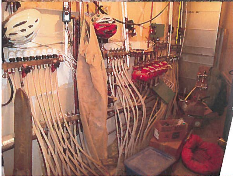
Distribution system in shop/guest house.
