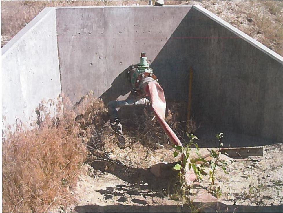
63-31688 License Exam 7/28/2011 Photo #4: Fill station close up. Outlet of buried 8" dia line from underground storage tank next to well.
