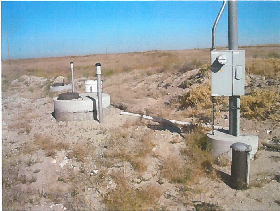
63-31688 License Exam 7/28/2011 Photo #2: Well (POD), power meter, and covers above 15,000 gallon underground storage tank facing west/northwest.
