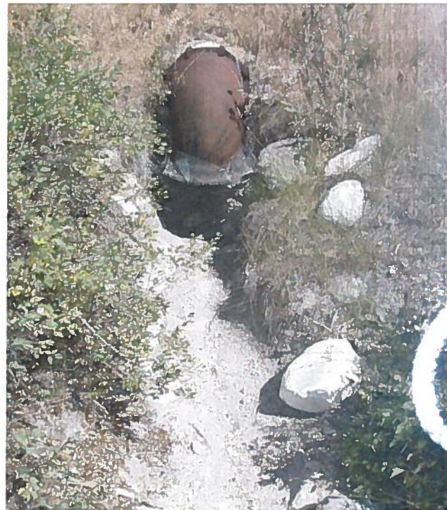
Photo #29 Well Overflow
