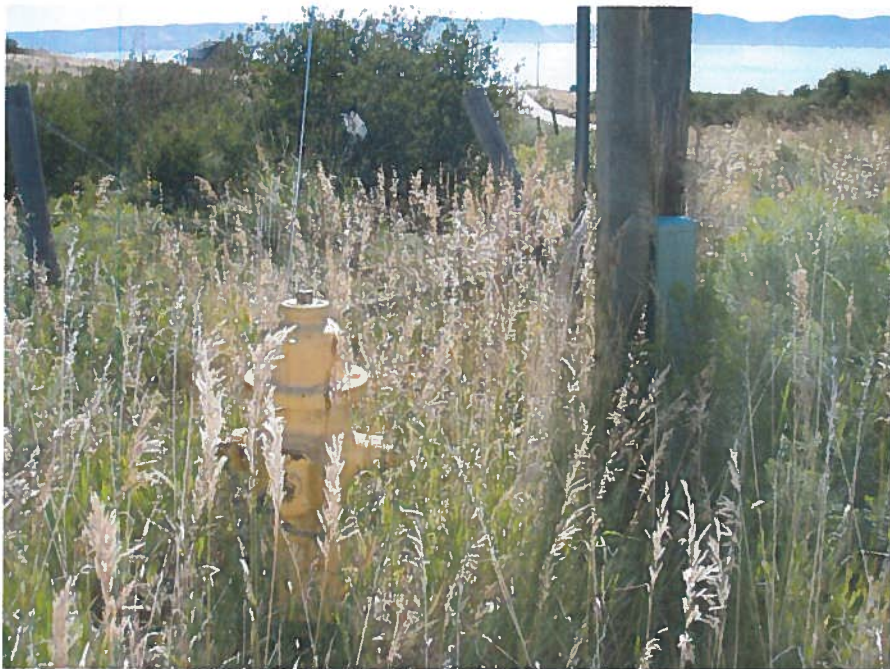
Photo #7 Example of a System Fire Hydrant
