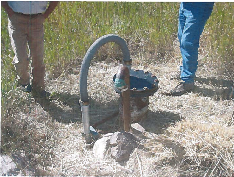
Photo #5 Well #1 & Vent
