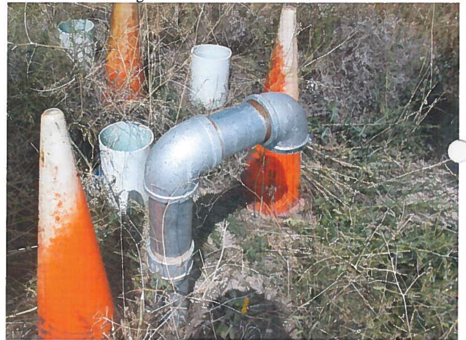
Photo #8 Pump to Waste Valves & Connection
