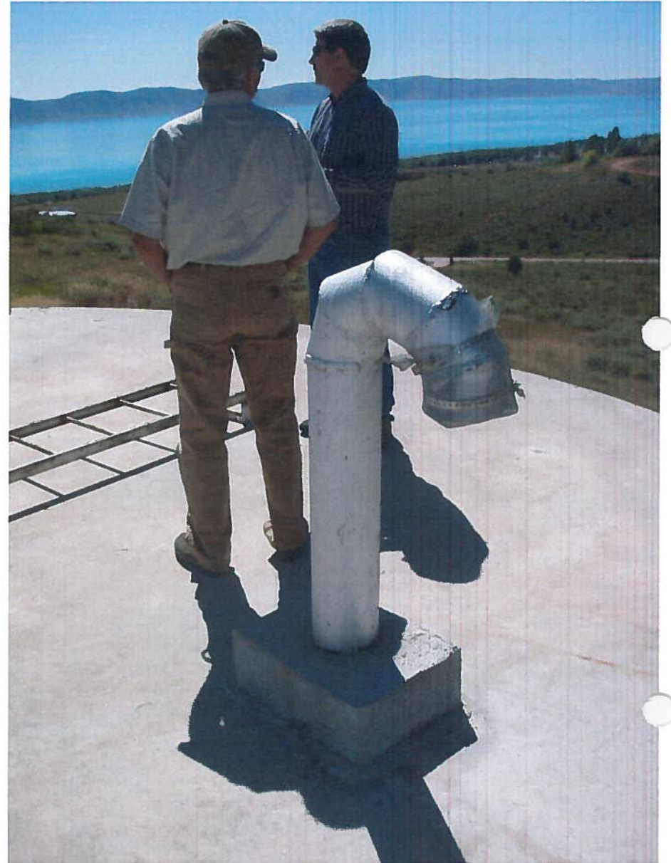
Photo #25 Screened Tank Vent and Access Ladder
