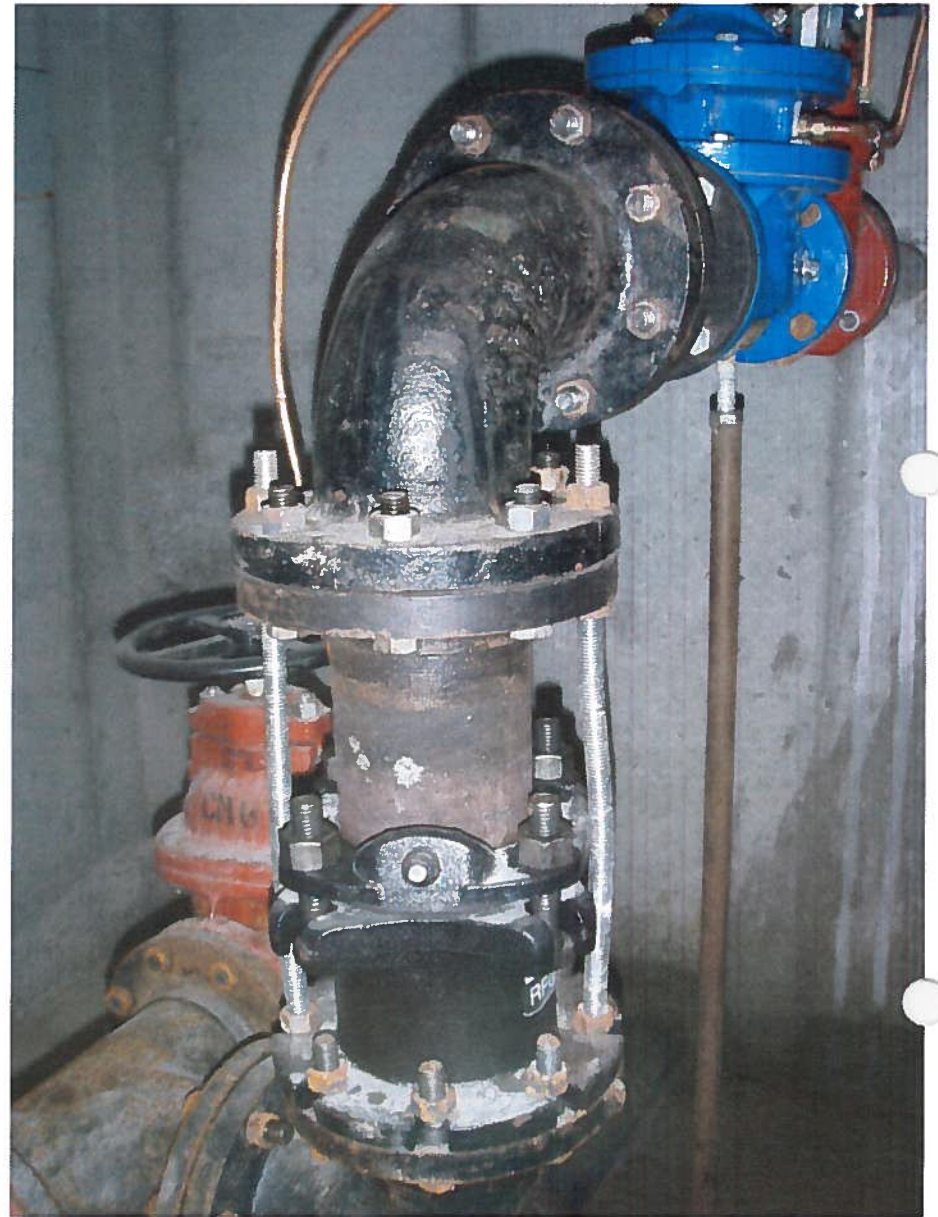
Photo #14 Distribution Piping Connections Well #1
