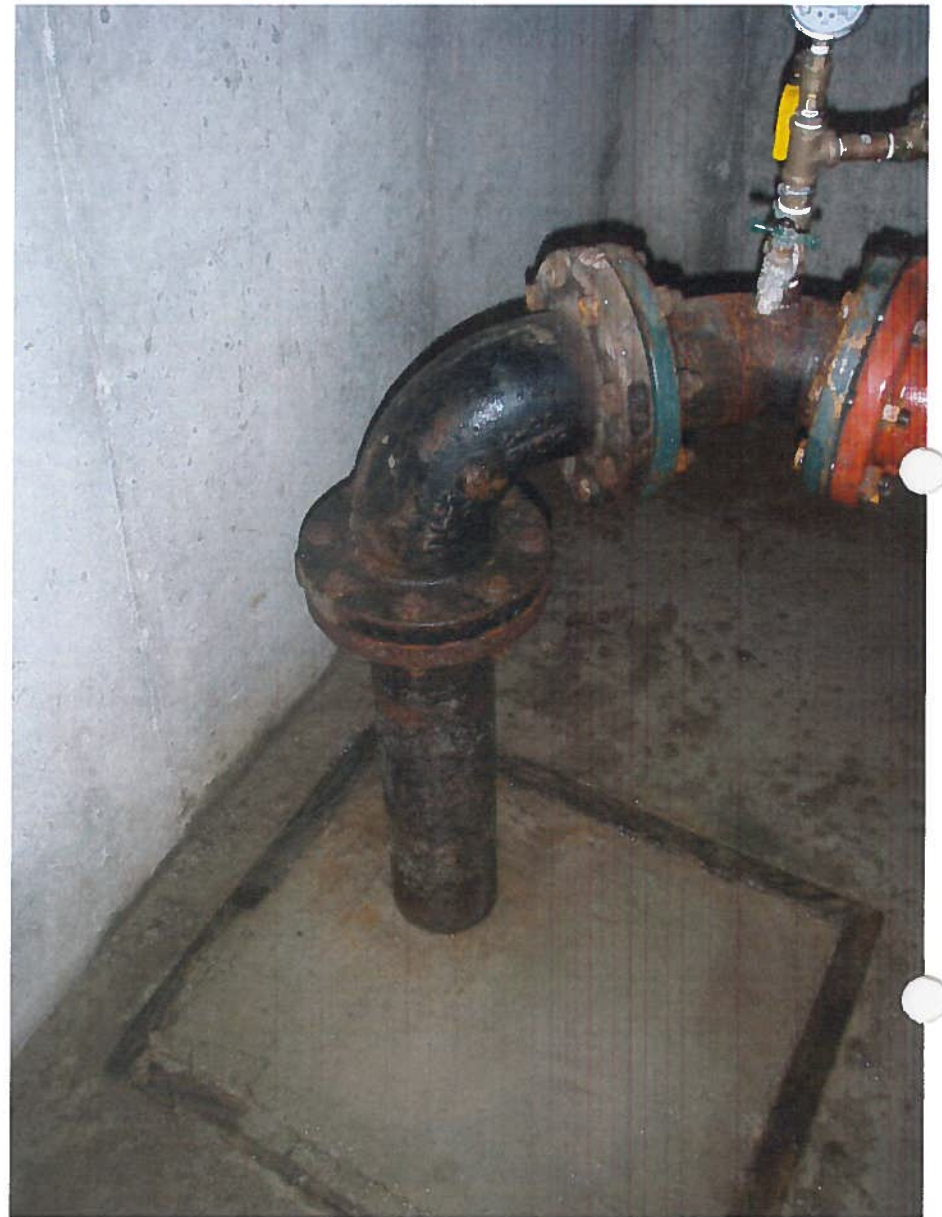
Photo #11 Piping Out to Distribution, & Sample Tap
