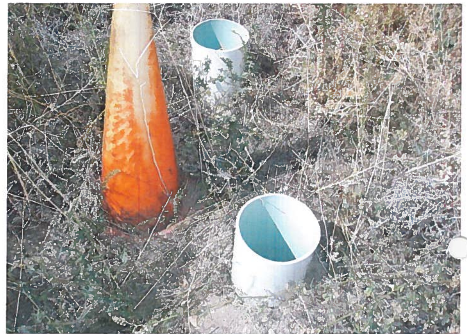
Photo #16 Distribution System Valves
