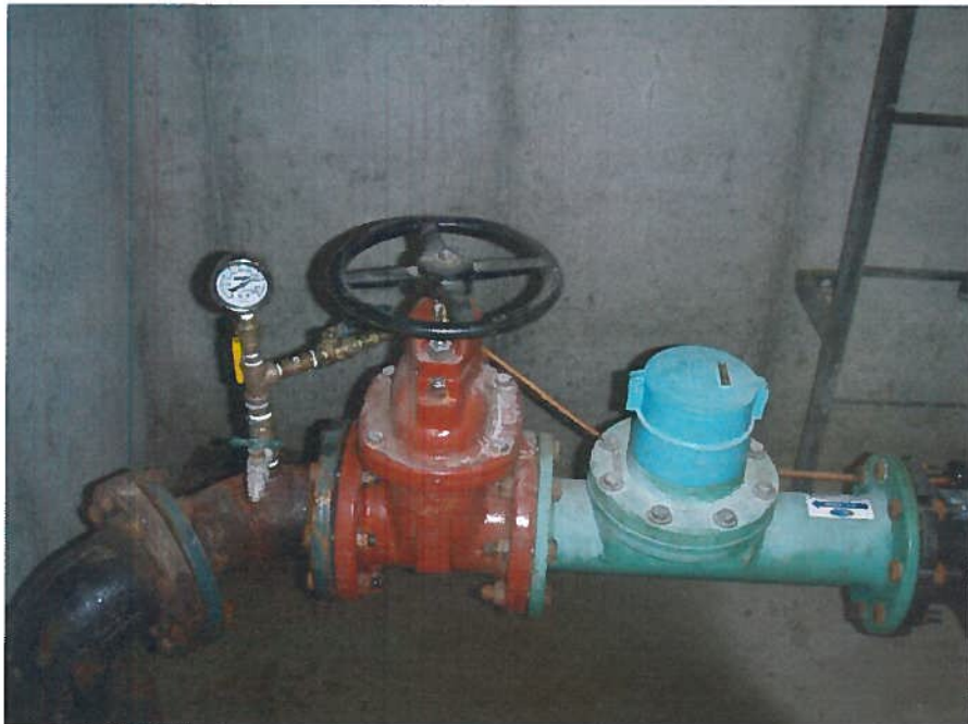
Photo #13 Isolation Valve, Pressure Gauge, Sample Tap, Flow Meter
