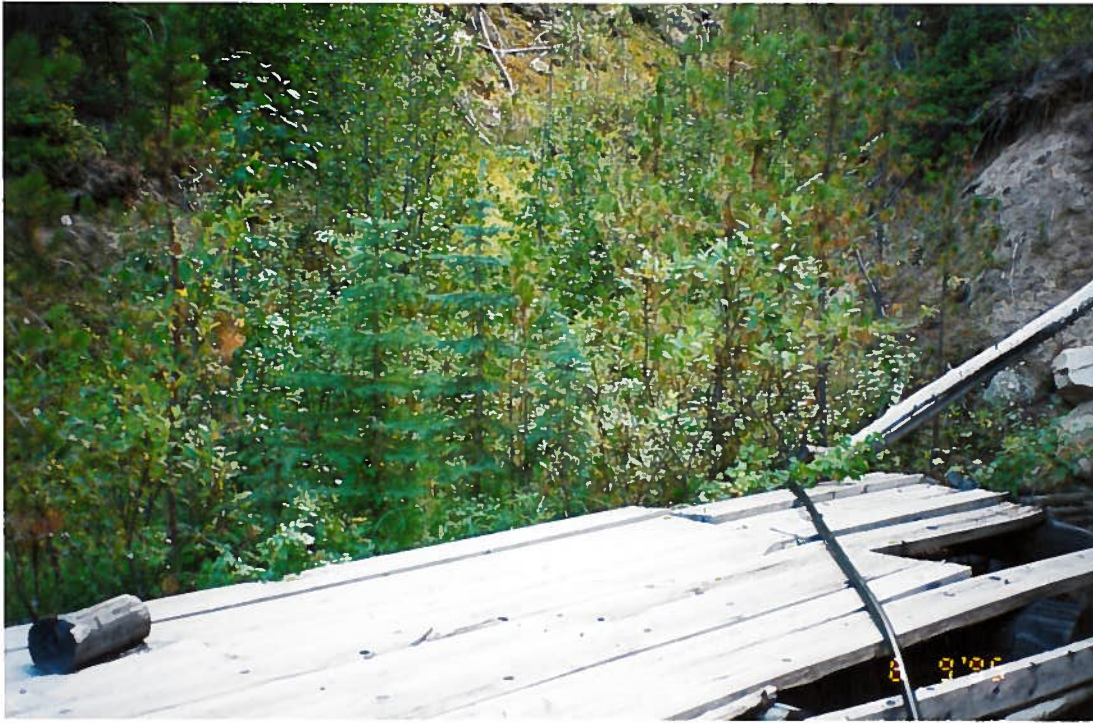
77-7310 Field Exam 9/6/1995 Photo #1: P/D pipe emerging from heavy brush at “Troll Tunnel”.
