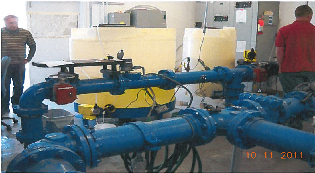
Inside pumphouse. Flowmeter gauge seen middle of photo. Water is pumped through 6" pipe up to piping seen in middle right and then underground [middle left] to reservoir . Piping in front of picture is from reservoir to booster pumps.
