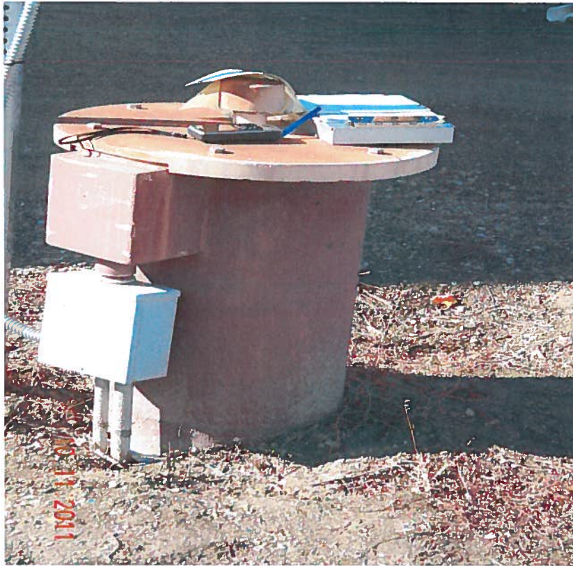
Well # 4. Drilled to 595' and filled with bentonite from 295' to 595'. 10" diameter. Screened from 205' to 235'. Submersible pump – specs of pump and motor unknown.
