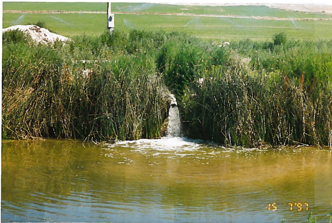
10" waste water discharge pipe into pond
