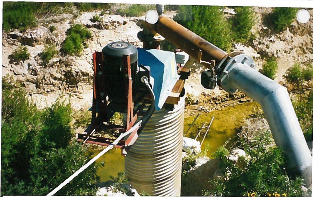
15HP Sump pump on WW drain
