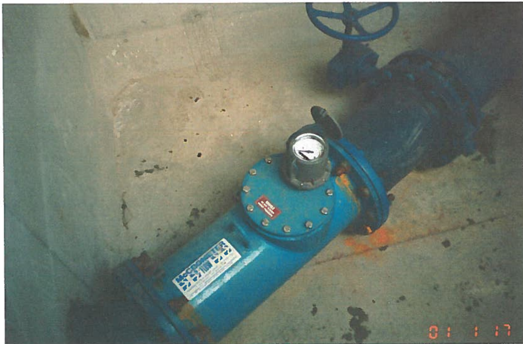
McCrometer 10" Flowmeter in 10" discharge line from well.
