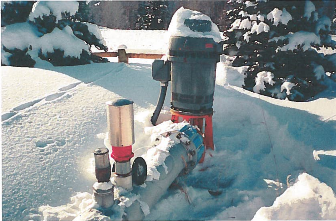
60 Hp Well Pump & Motor - Discharges to 10" steel line prior to going underground.
