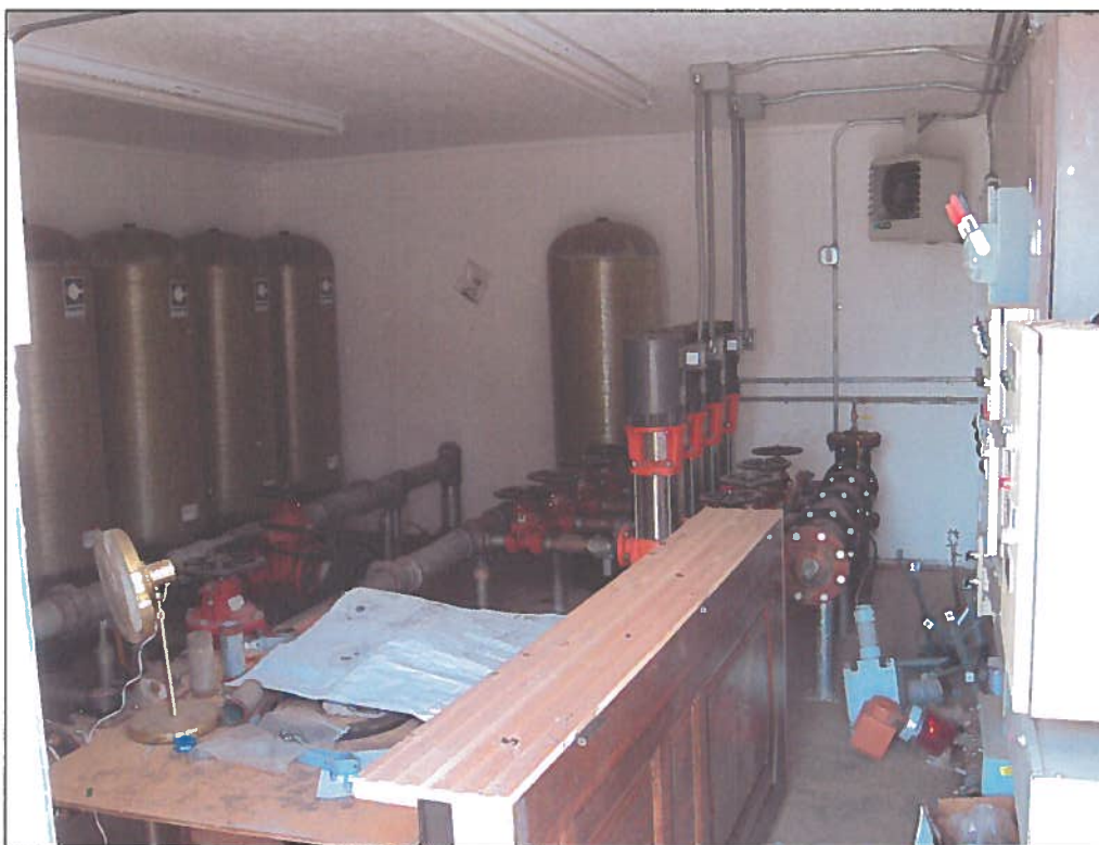
Photo 8: Municipal potable water booster station pumps, pressure tanks, controls, and mechanical piping.
