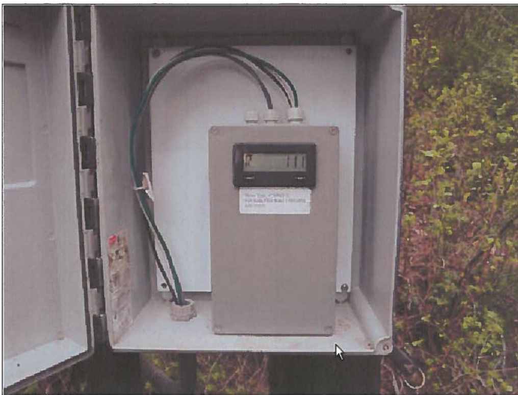
Photo 9: Well #4 flowmeter display (111 gpm).
