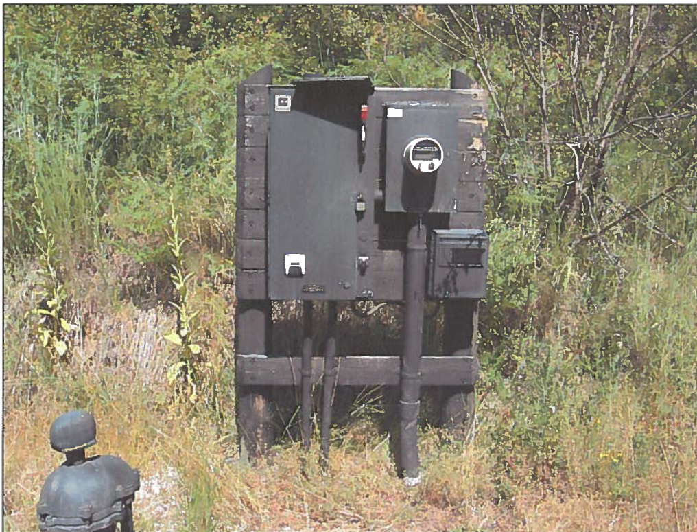
Photo 6: Well #9 main power panel.
