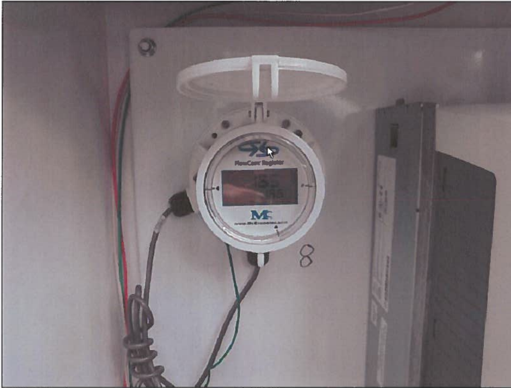
Photo 11: Well #8 flowmeter display (165 gpm).
