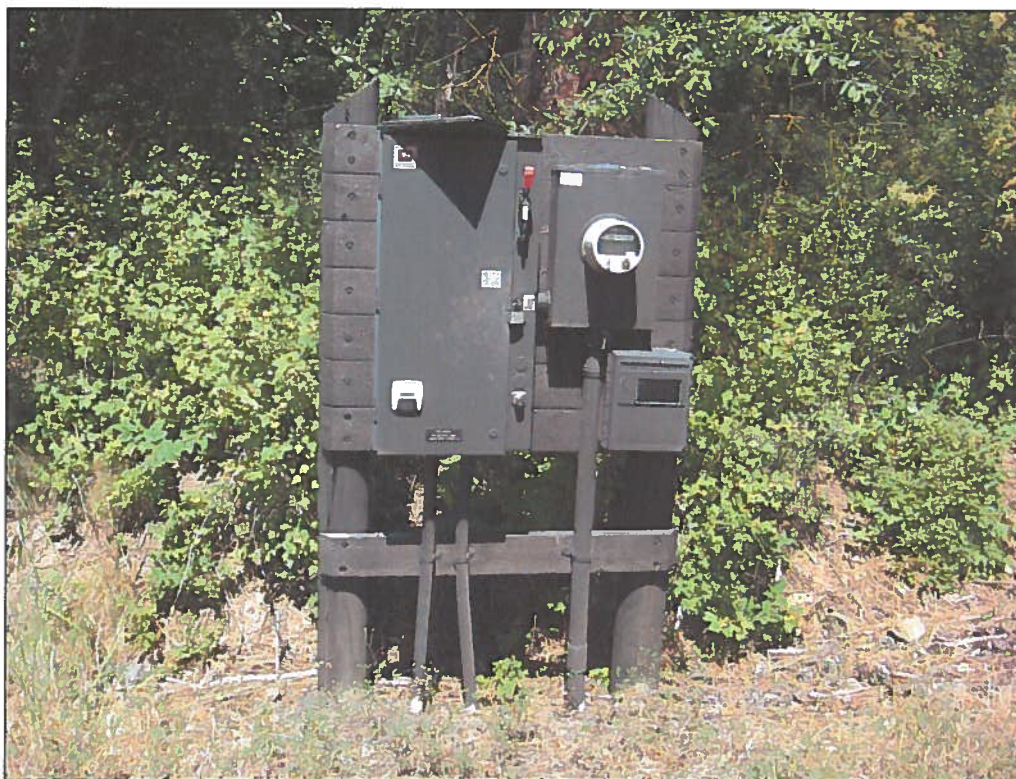
Photo 2: Well #4 main power panel.
