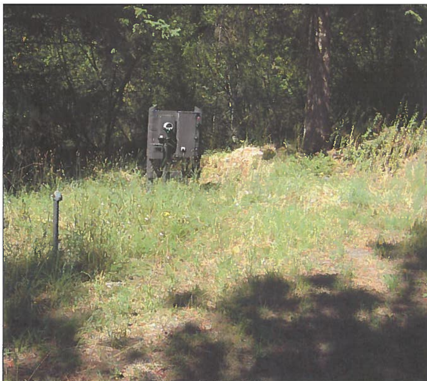
Photo 4: Well #8 main power panel.
