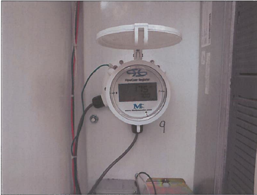
Photo 13: Well #9 flowmeter display (175 gpm).
