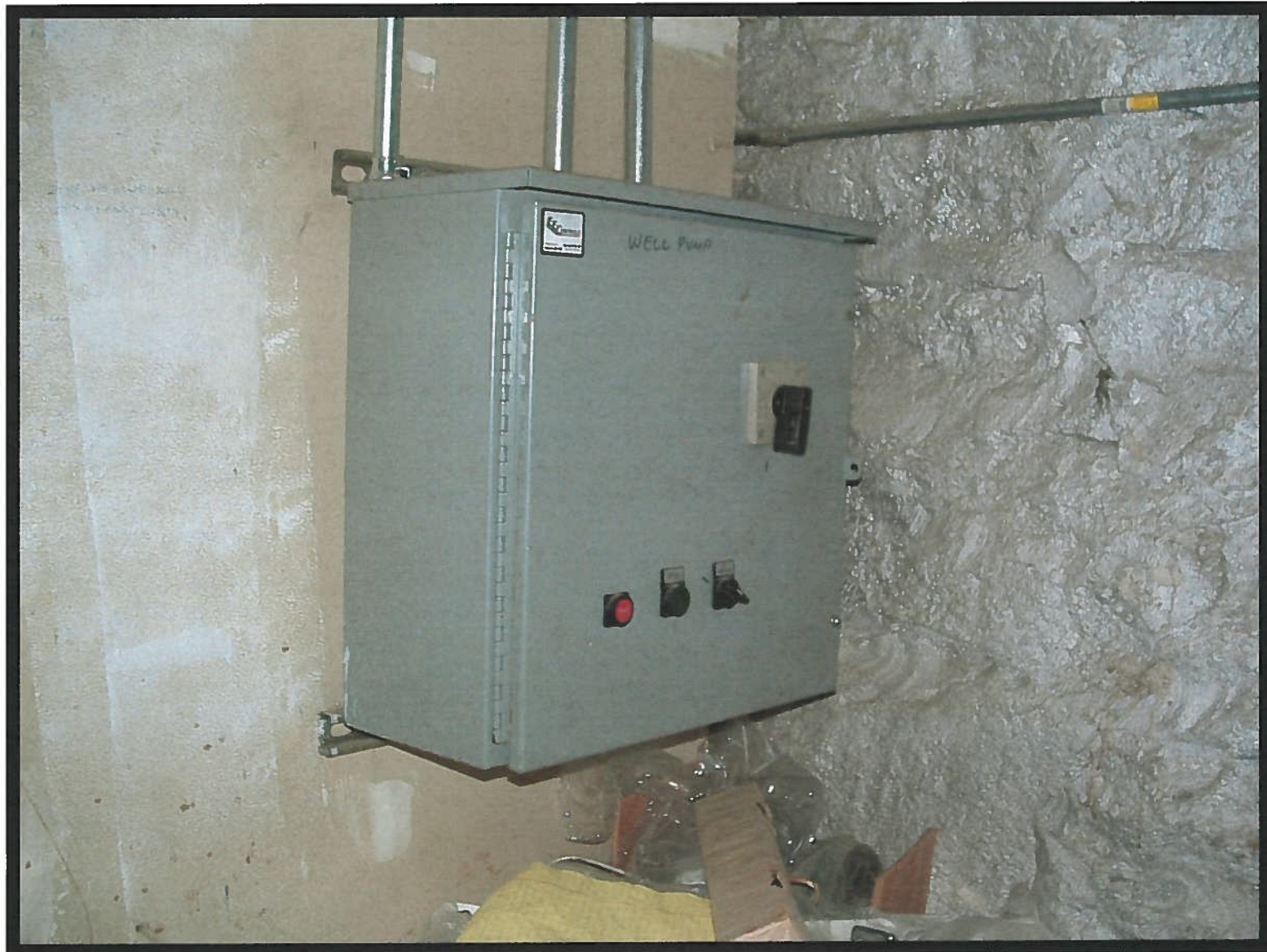
Well Pump Panel
