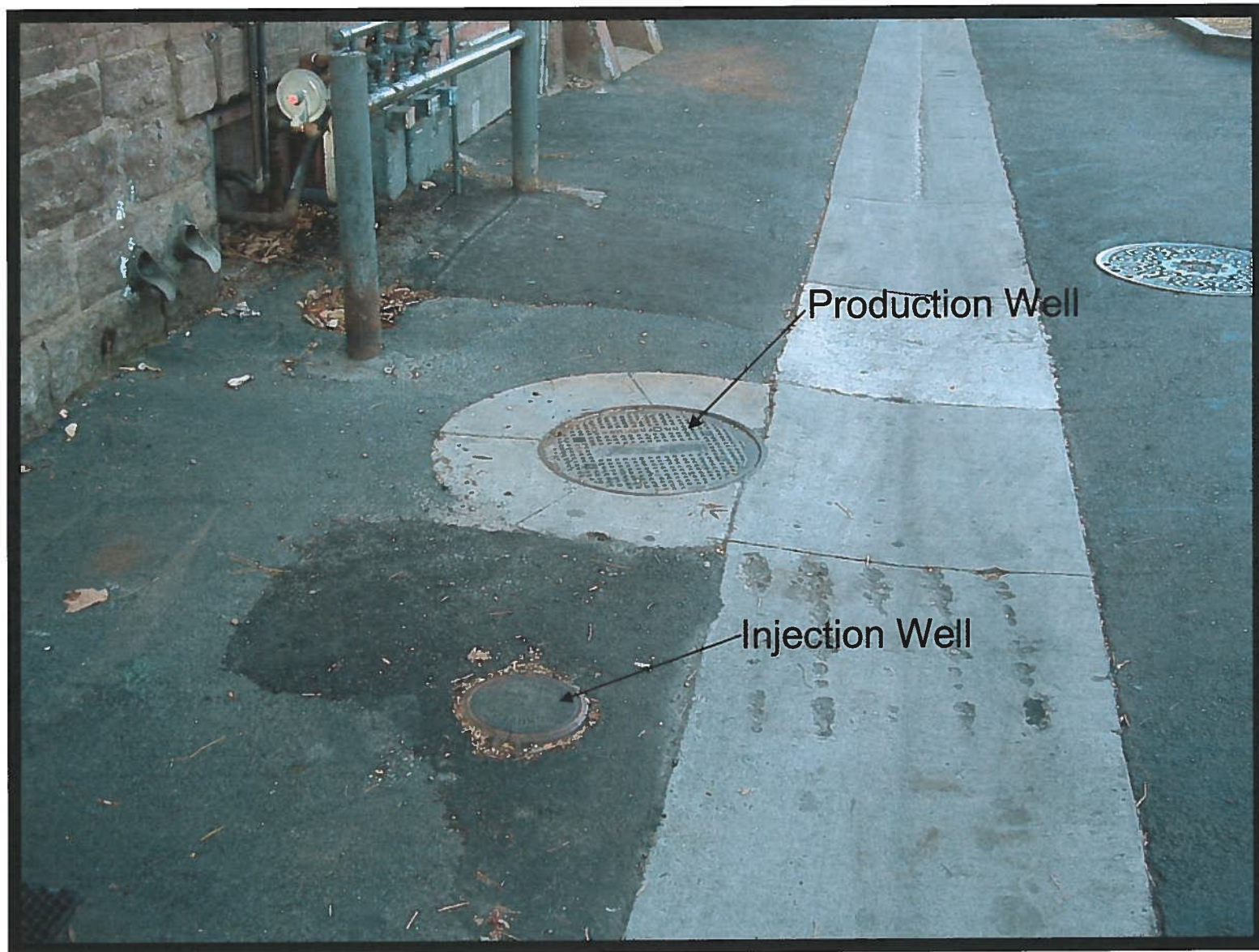
Point of Diversion and Injection
