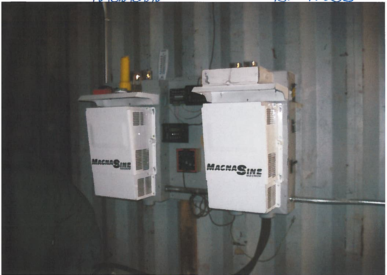
AC Converter Boxes
