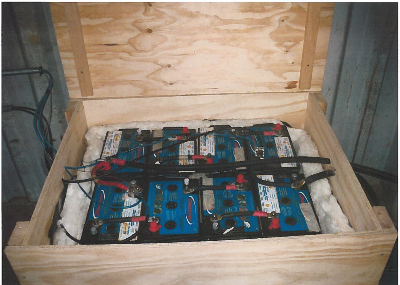
Battery Storage Unit
