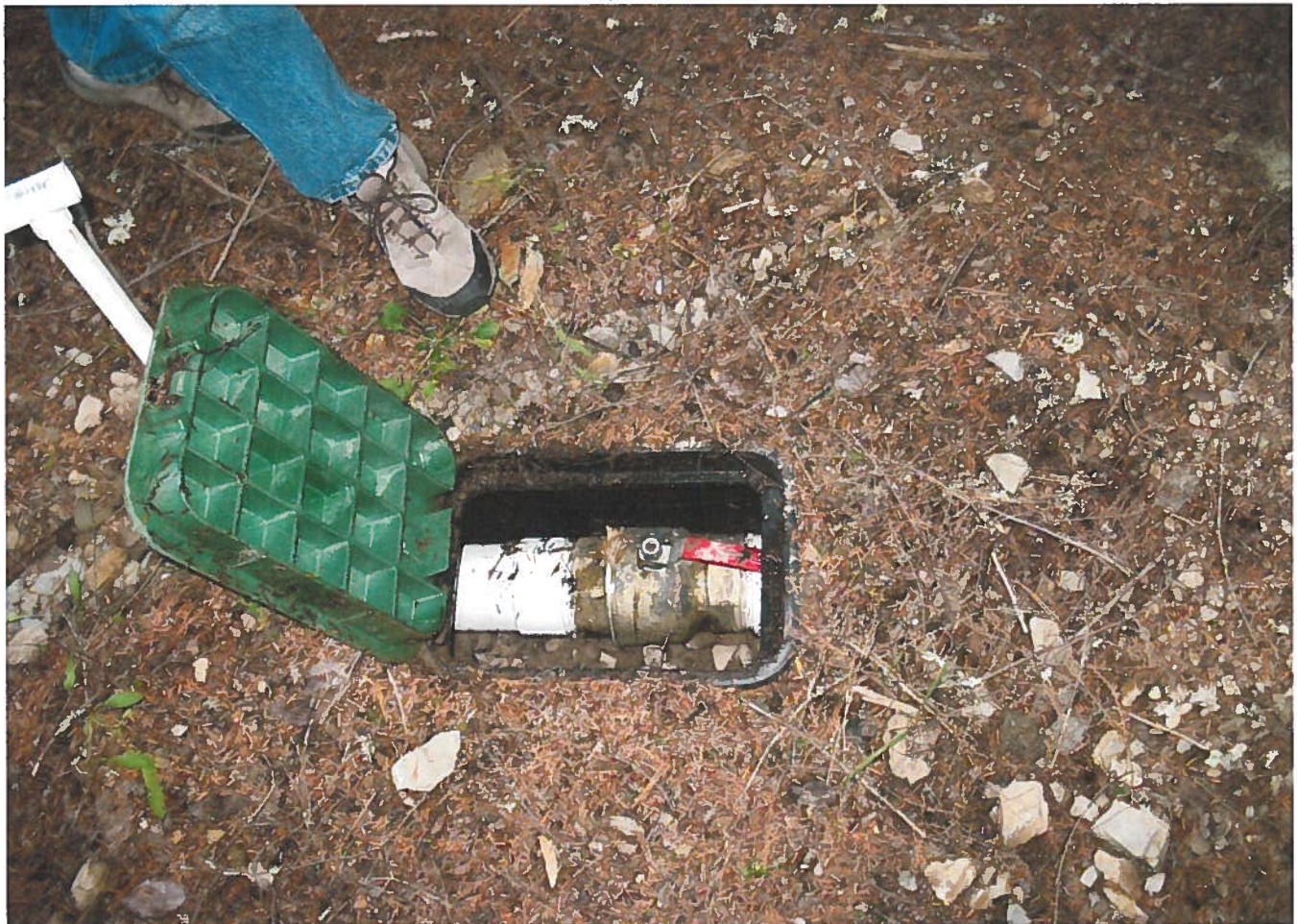
Penstock shut off valve
