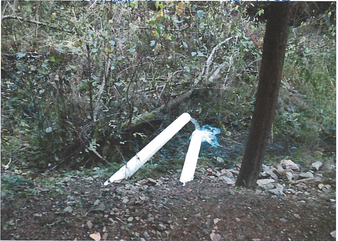
Emergency Over Flow From Cistern
