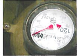
Flow- Well 98-93-N-0021.JPG
