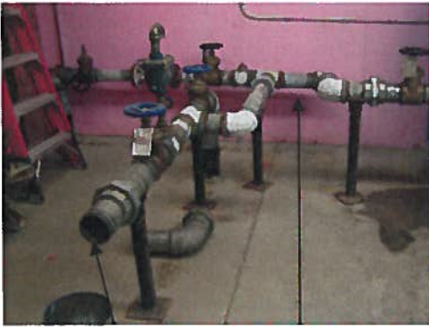
Pump to waste
