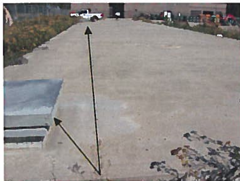
Reservoir with access risers
