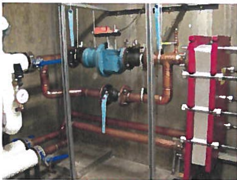
Heat exchange system
