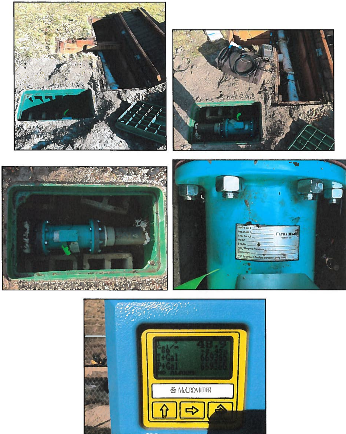
Figure 2. Johnson Ranch wells meter installation and meter reading on 12/12/2011.
