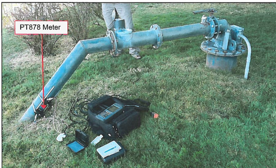
Figure 4. PT878 meter installation at Well No. 3.
