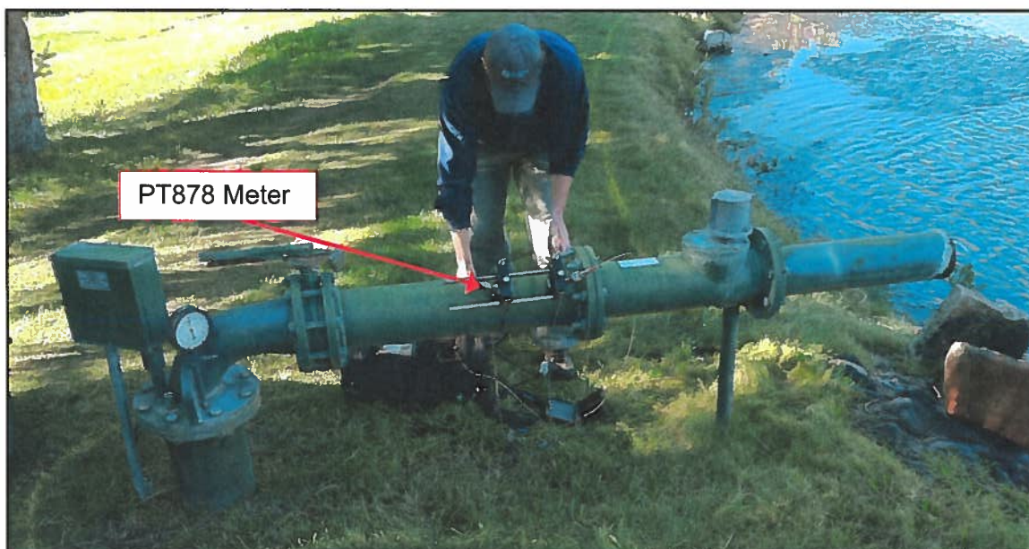
Figure 3. PT878 meter installation at Well No. 2.
