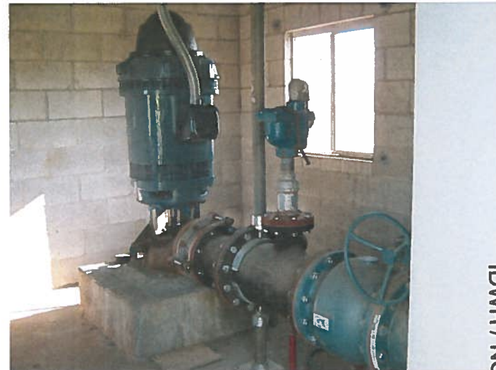
Well No. 2 and Vertical Shaft Turbine Pump
