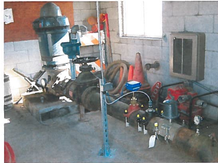
Well No. 1 and Vertical Shaft Turbine Pump
