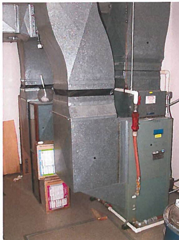
Figure 2: Heat Pumps & Ducting
