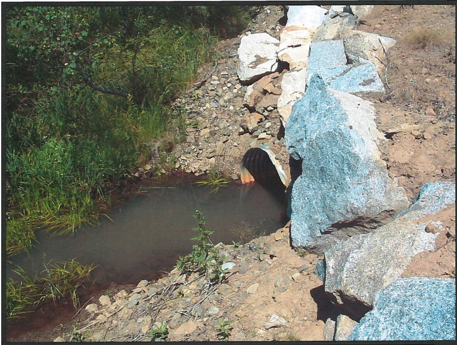
Unnamed Stream Bypass Culvert Outlet
