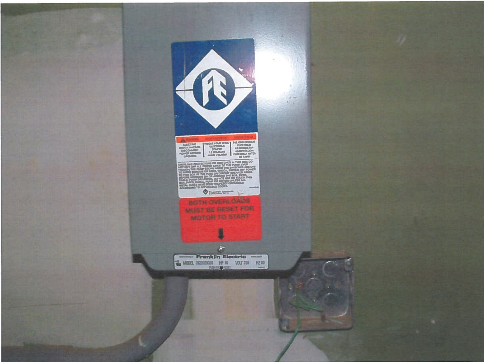
Well No. 1 Control Box
