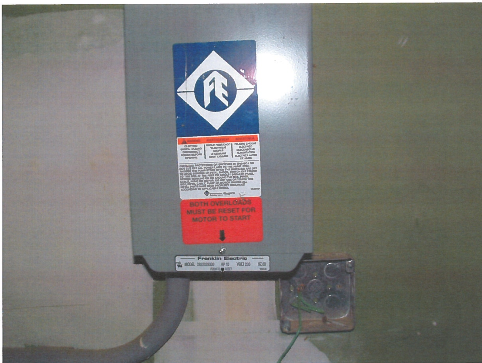
Well No. 1 Control Box
