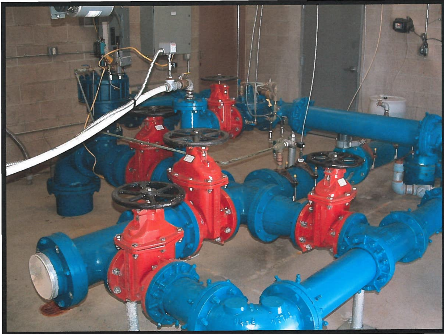
Well house piping
