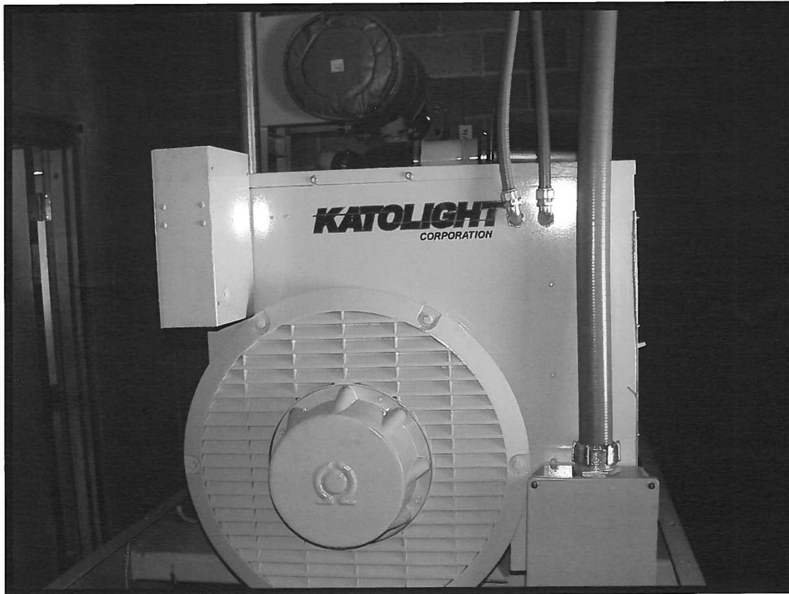
Back-up power generator
