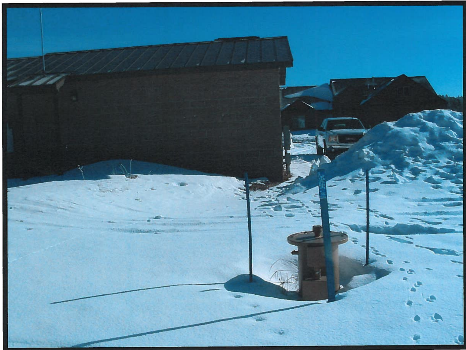
16-inch well (pitless unit in foreground; well house in background)
