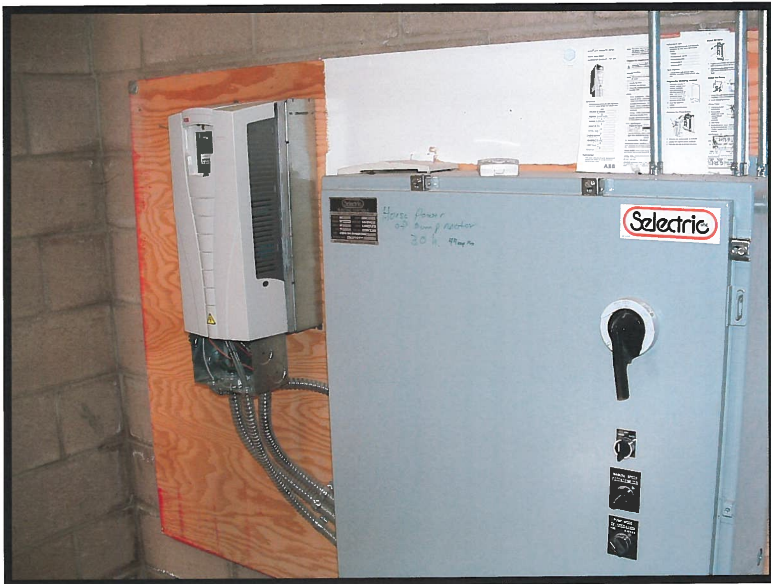
30-hp pump panel and vfd
