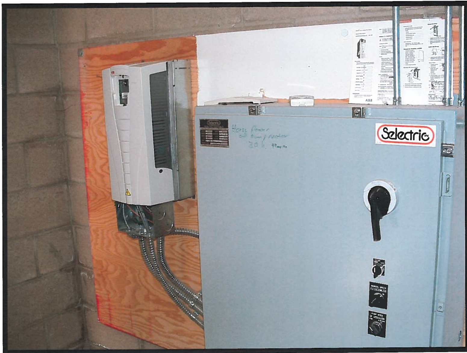
30-hp pump panel and vfd
