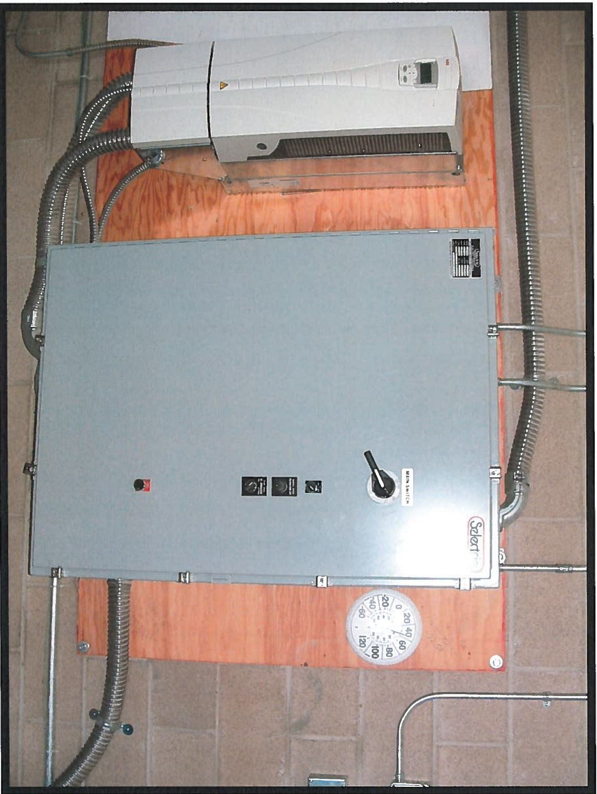
100-hp pump panel and vfd
