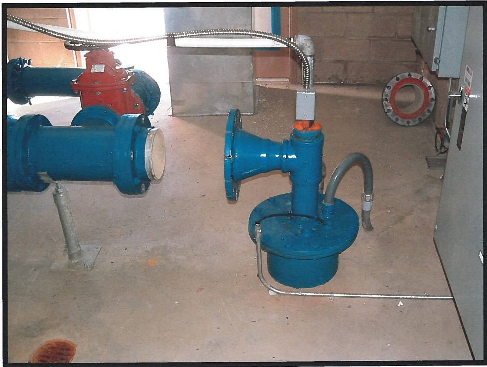
12-inch well (30-hp pump disconnected for service; 1 hp pump active)
