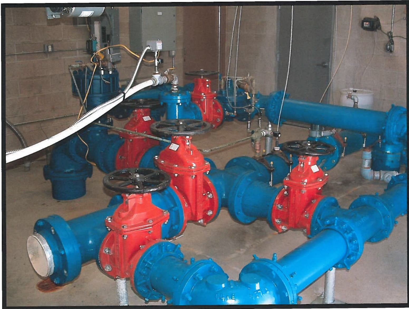
Well house piping
