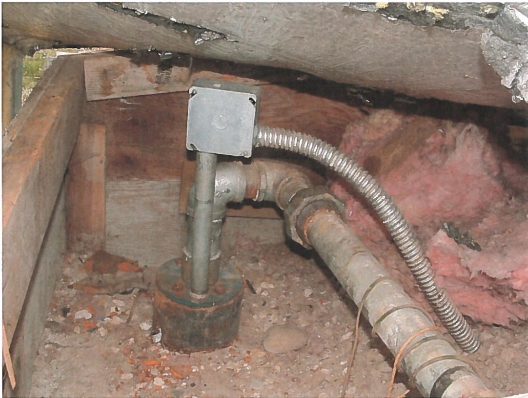
Point of diversion - well head in shelter on south side of well house
