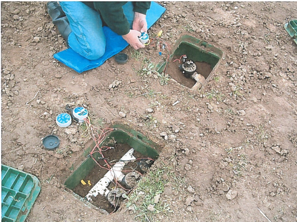
Pasture sprinkler valves
