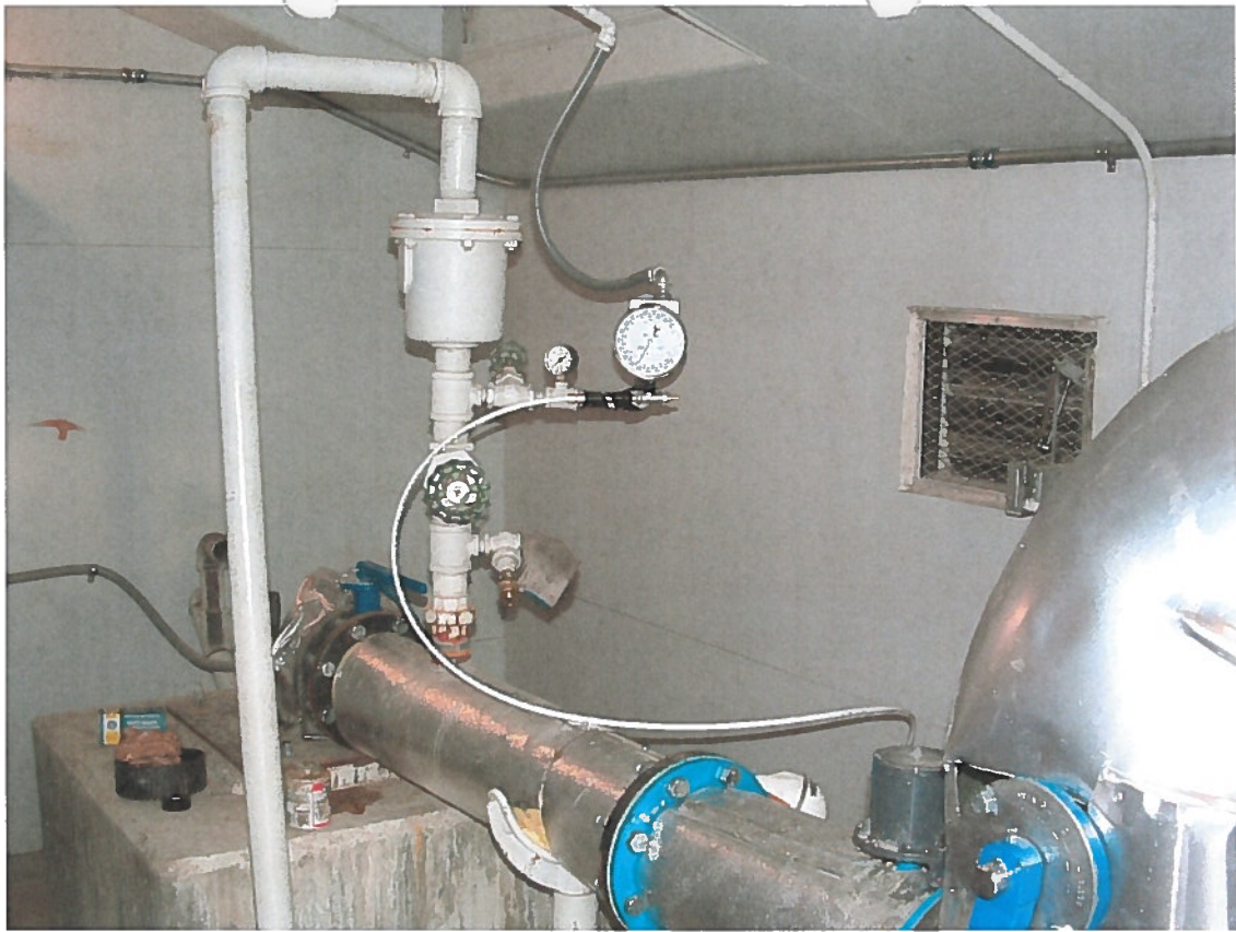
Well 1 - well head and discharge piping (Well 1 well house)
