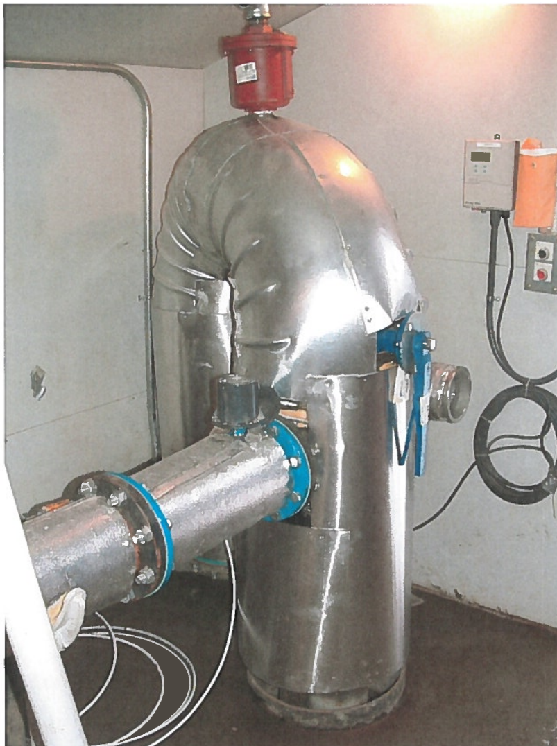
Well 1A discharge piping (at Well 1 well house)
