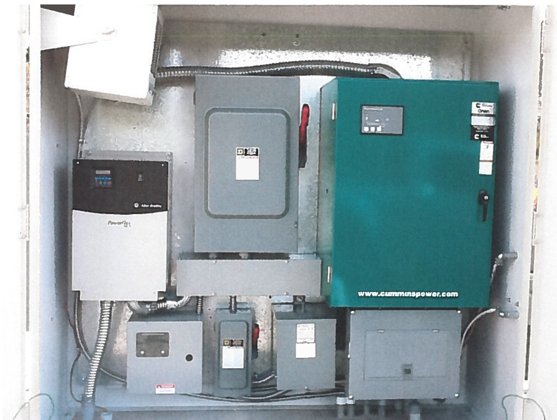
Well 5 Panel (VFD, autotransfer switch, disconnect)
