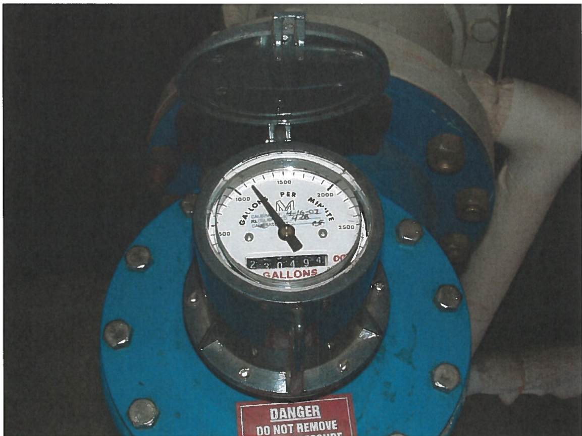
Well 3 Flow meter
