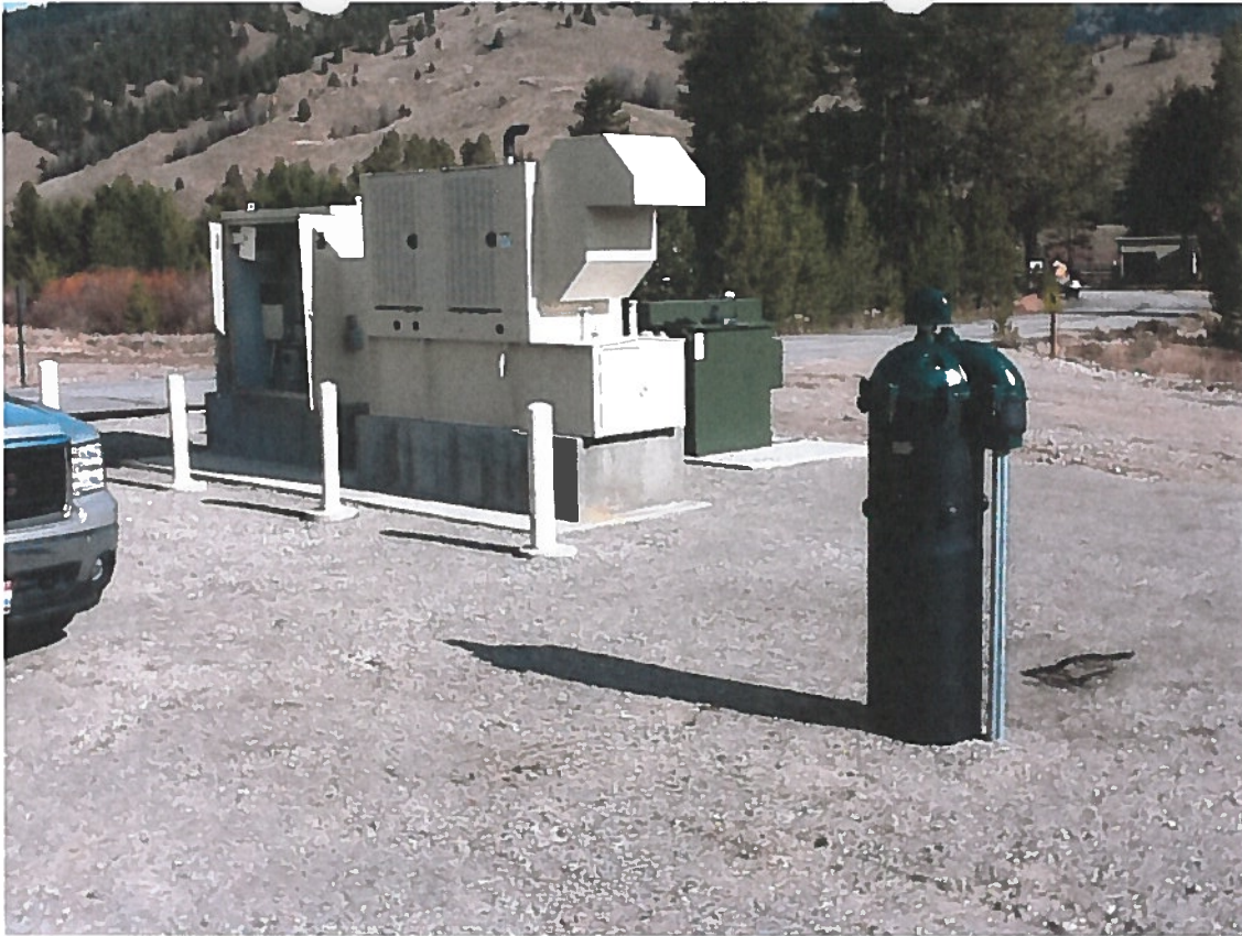
Well 5 (foreground) with generator, panel, and transformer
