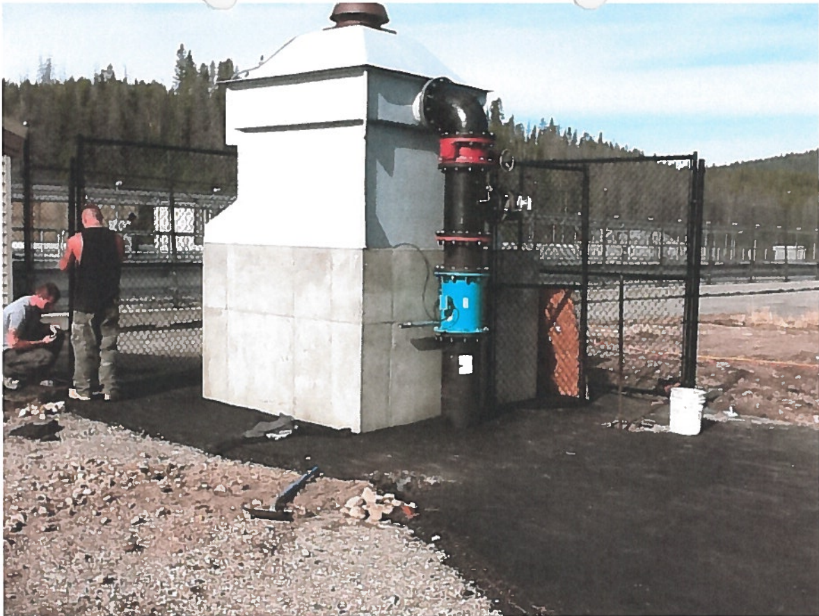
Well 5 Discharge to adult holding degas facility; flow meter is blue-green spool
