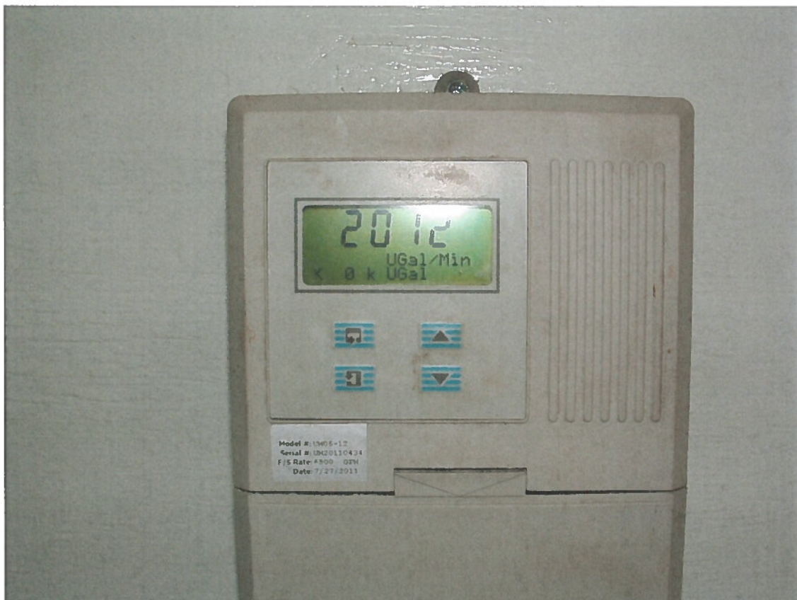
Well 5 Flow meter Display (at raceway degas building)
