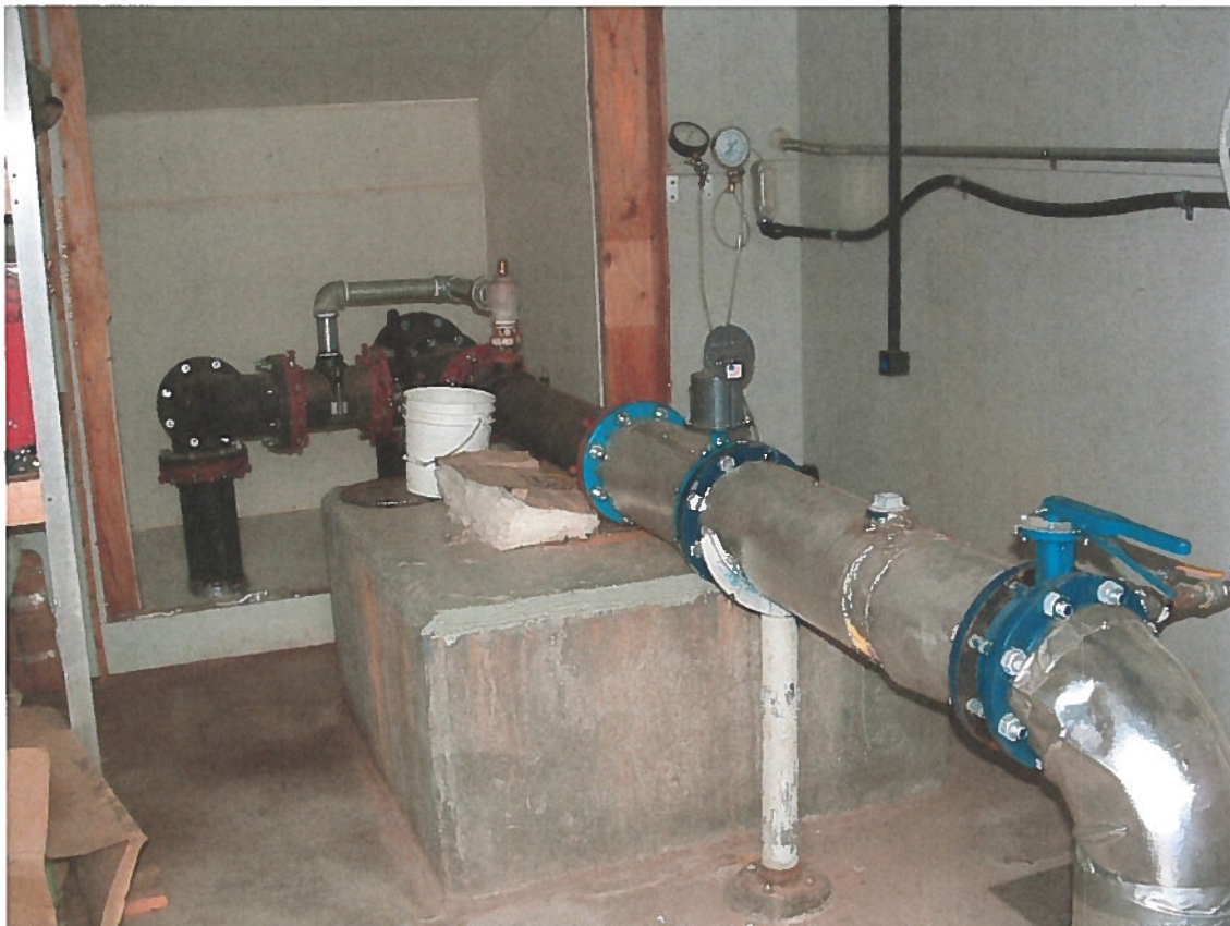
Well 6 and 7 discharge piping in Well 6 & 7 well house (former Well 2 well house)
