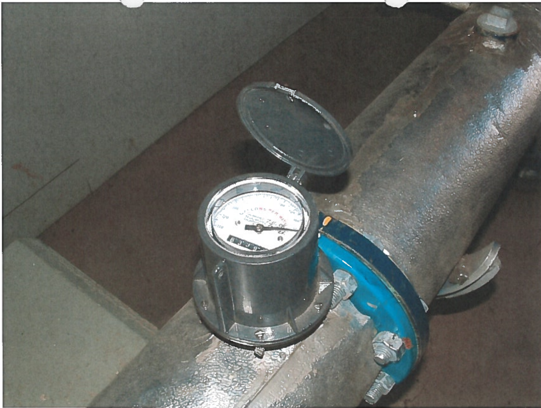
Well 6 and 7 flow meter in Well 6 & 7 well house (former Well 2 well house)
