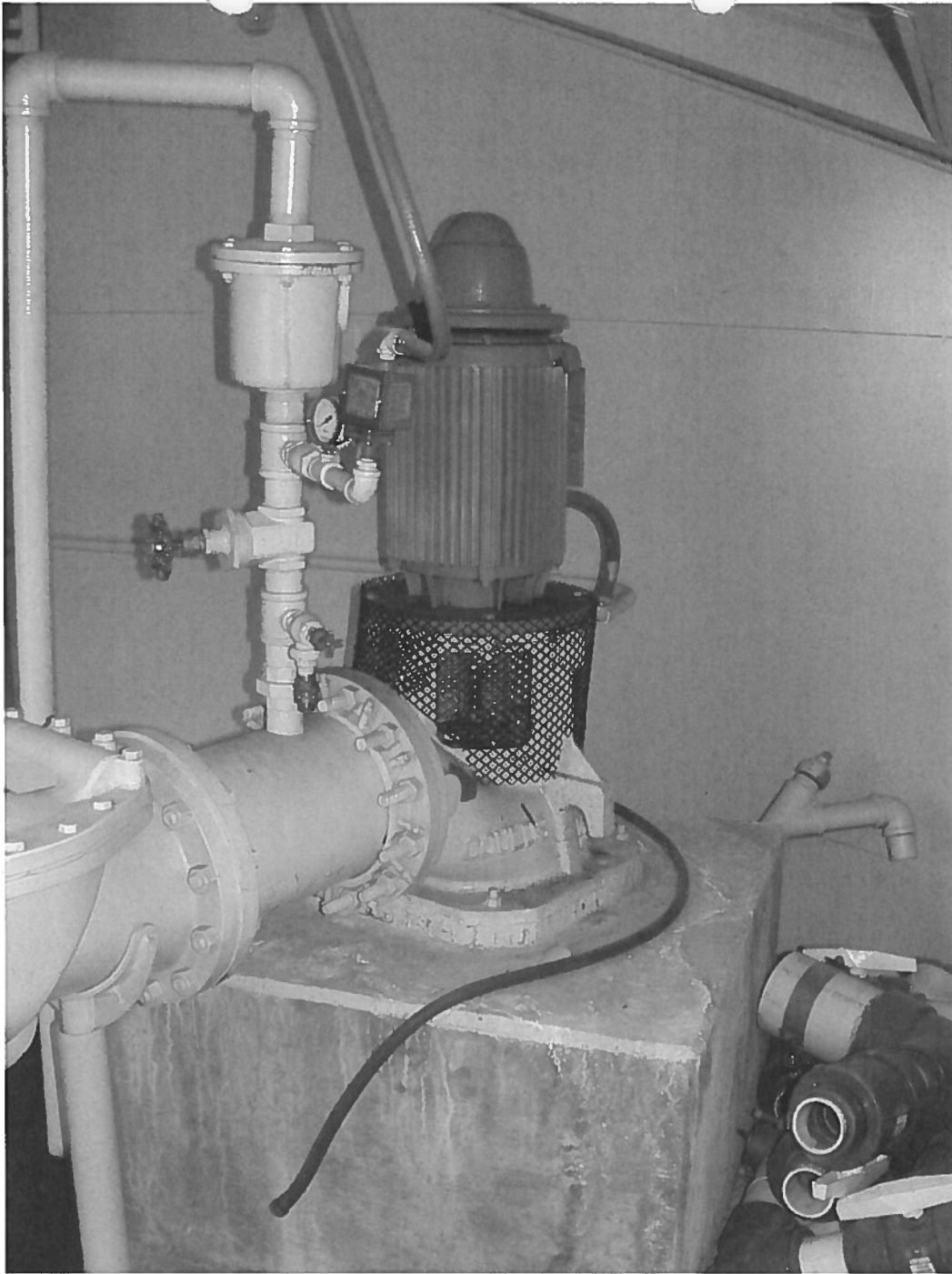
Well 3 well head (in Well 3 well house)
