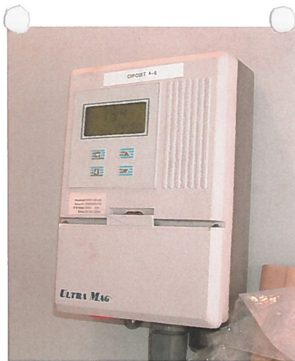
Well 1A flow meter display (at Well 1 well house)
