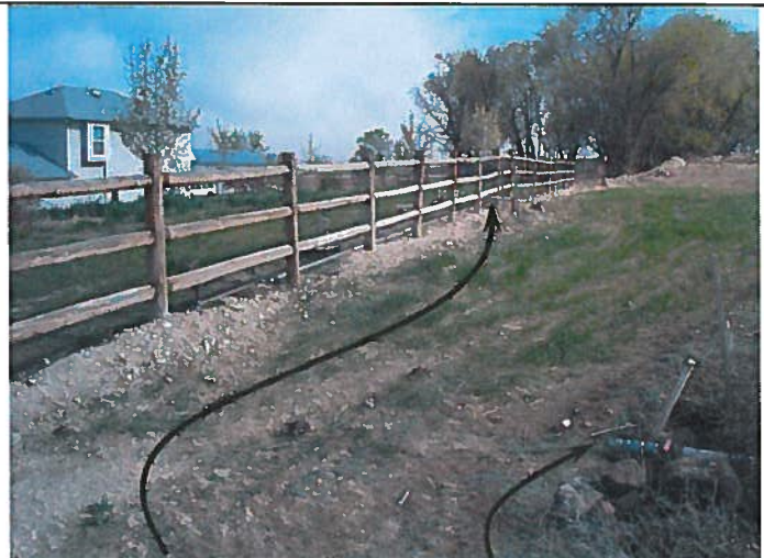
Mainline connection To pasture system canal tap
