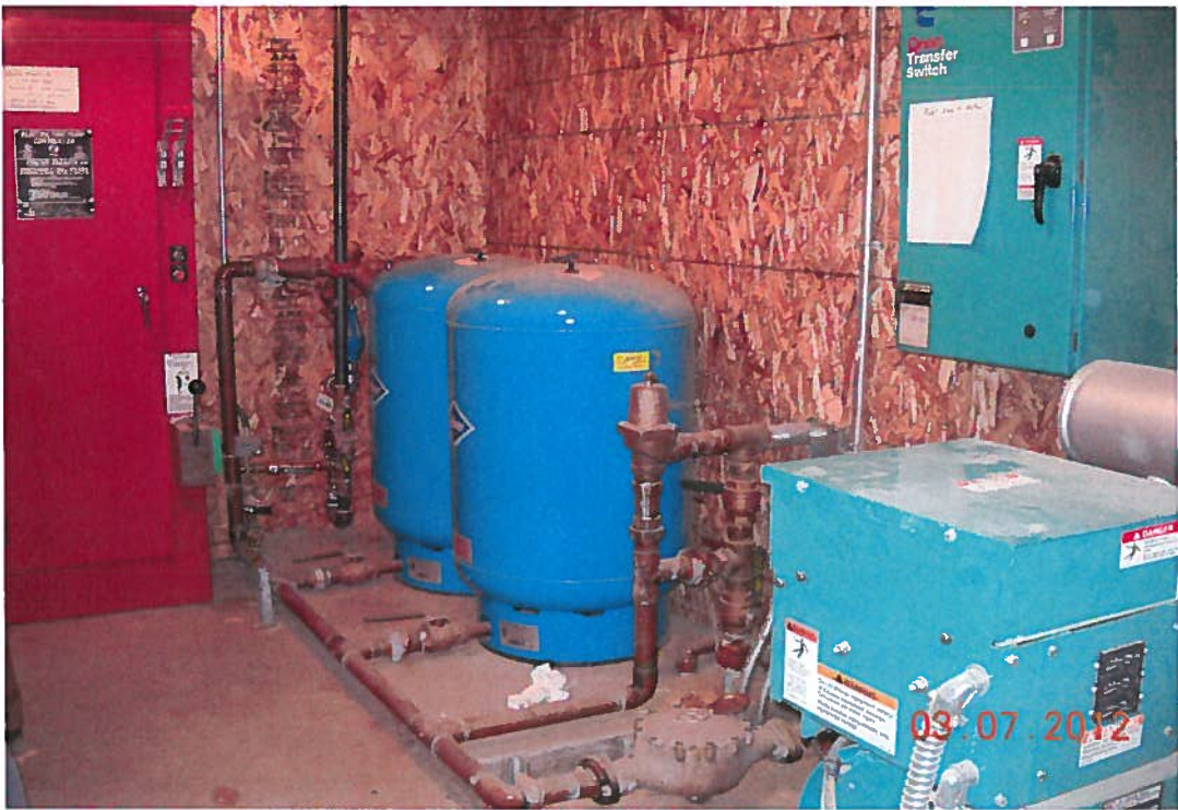
Looking southeast at the domestic system inside the well house.
